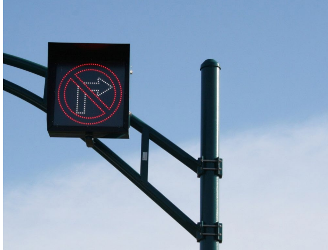
Figure 3: LED Blank-out Sign ( source: Orange Traffic )
