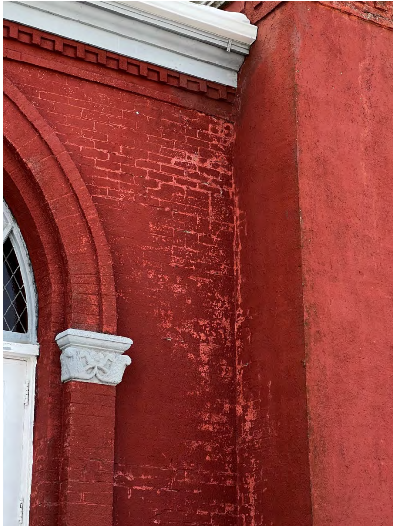
Figure 41e: St. Mark's Church, 5522 Russell Street (connection between entry wall and north tower)
