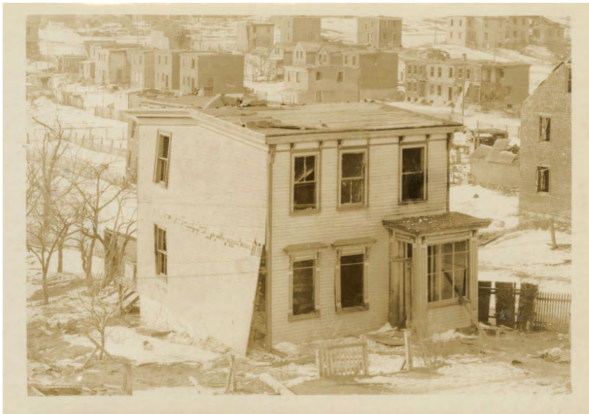
Figure 10: 510 Gottingen Street, corner of Gottingen and Livingstone Streets Source: W.G. MacLaughlan Nova Scotia Archives 2014-031
