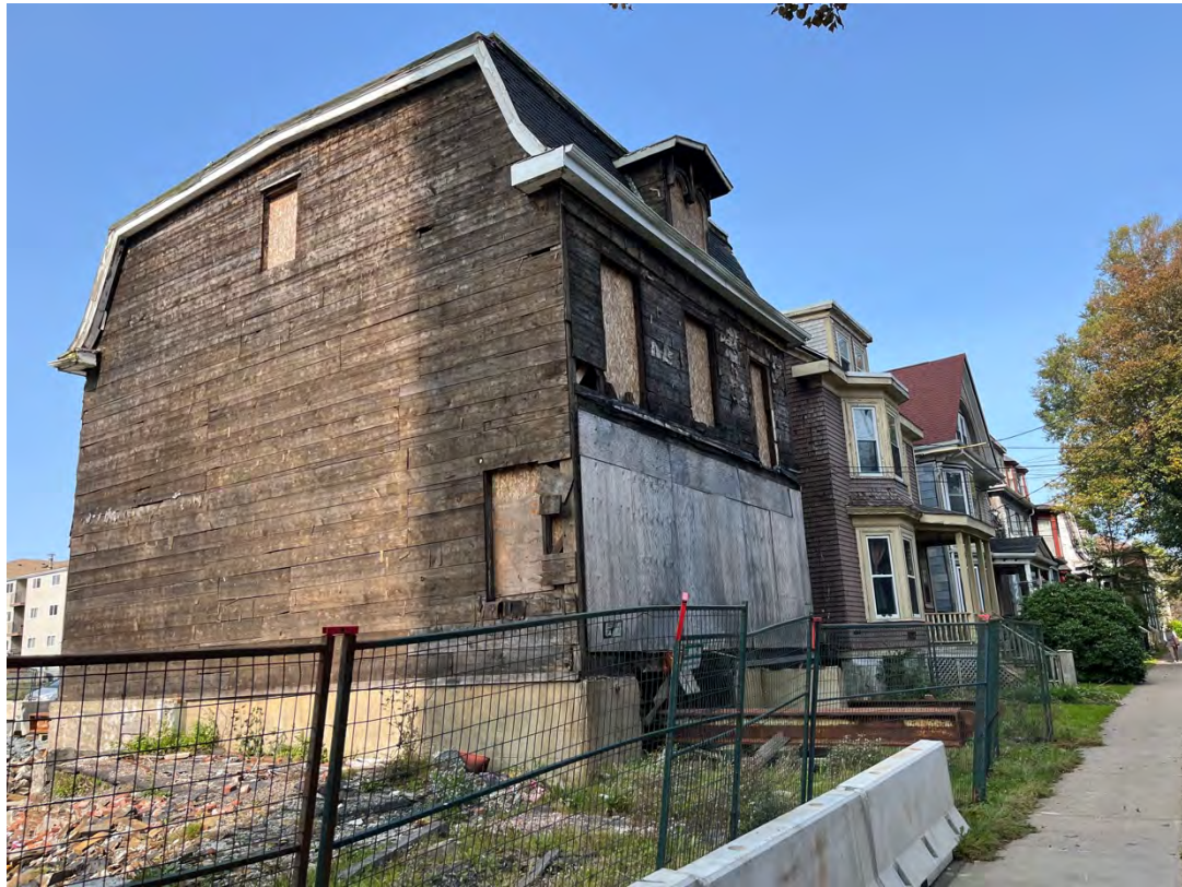
Figure 33: 1456 Carlton Street following unauthorized alterations (front and south side)
