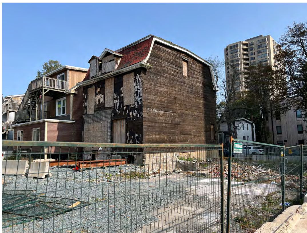
Figure 34: 1456 Carlton Street following unauthorized alterations (rear and south side)
