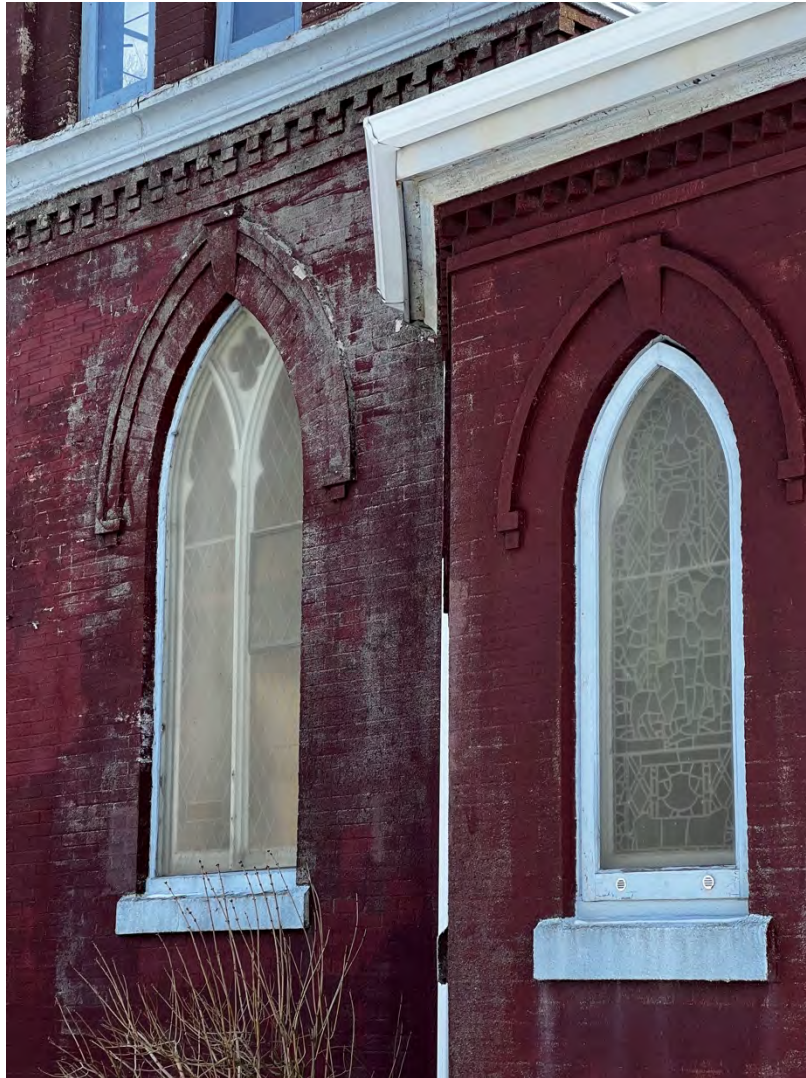
Figure 41k: St. Mark's Church, 5522 Russell Street (connection between base of north tower and protruding alcove)
