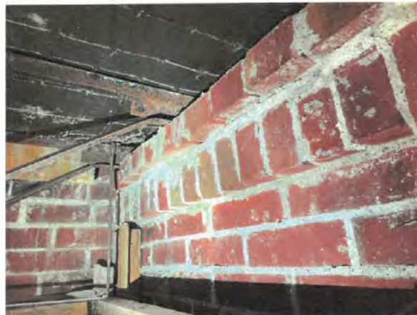
Photo No. 16 – Limited OWSJ bearing on brick corbel at exterior load bearing masonry wall – 1947 addition.
