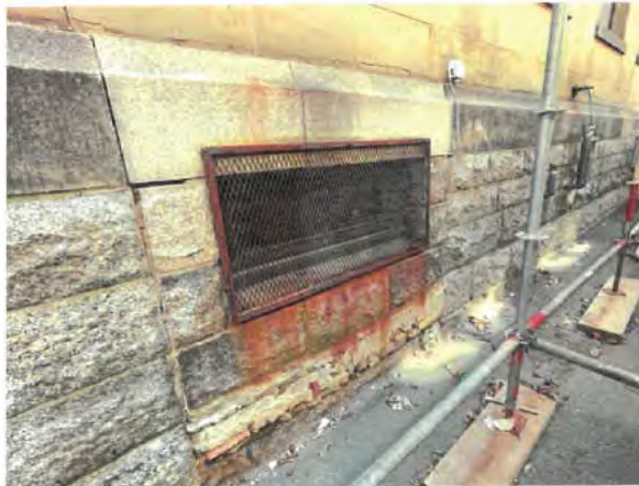
Photo No. 8 – Deteriorated joints and below sill infill at foundation wall opening.
