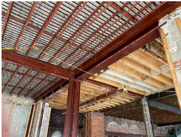
BMR Photo 5.3.A: Interface between 1961 addition to be demolished in foreground and original Post Office in background. Original load-bearing masonry and stone removed to create this opening (28 Feb 2022).
