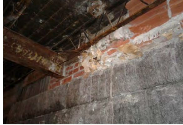
BMR Photo 4.6.F: Corroded steel floor joists and steel girder beam at 1947 addition. Recommend floor be demolished and replaced (1 Mar 2022).
