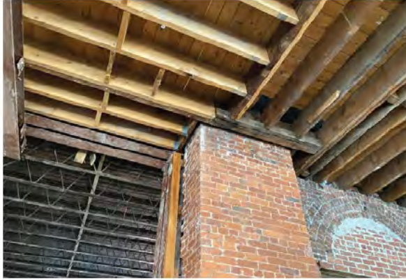
BMR Photo 4.4.A: Double 2"x12" timber header joist to be reinforced (28 Feb 2022).
