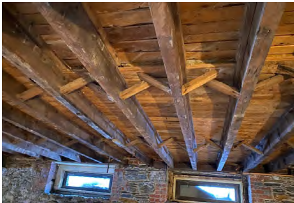
BMR Photo 4.6.A: 3"x12" floor joists with concrete infill between and cement terrazzo floor on top (1 Mar 2022).
