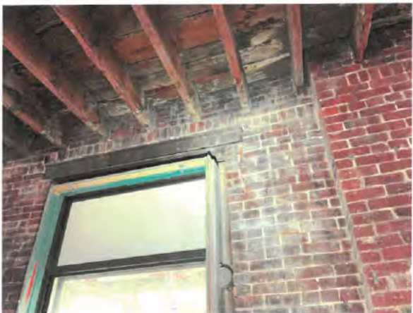
Photo No. 20 – Steel lintel over window with jamb brick cracking at window head. Note water staining of wood framing above.
