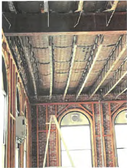
Photo No. 15 – Curved and out of plumb open web steel joists (OWSJ) in roof of 1947 addition.
