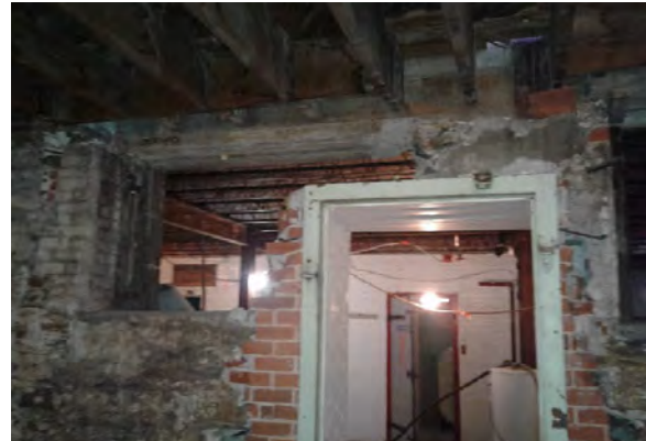
BMR Photo 4.6.D: Damaged load-bearing masonry and concrete infill with large column point load above door frame. Requires immediate attention (1 Mar 2022).
