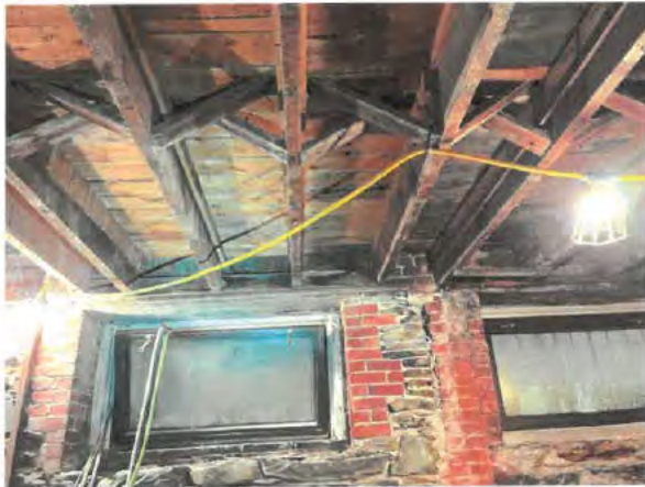
Photo No. 11 – View of 1914 main floor joists supported on wood lintel over window opening.
