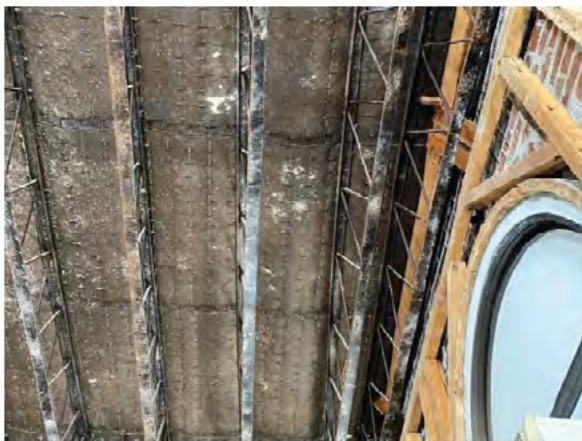
BMR Photo 4.4.E: Failed roof joists at 1947 addition shown buckled out of plane. No bracing or bridging present (28 Feb 2022).
