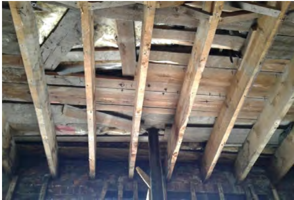
BMR Photo 4.2.A: 2"x10" timber joists with loose/damaged attic planks. Joists bearing on masonry wall (28 Feb 2022).
