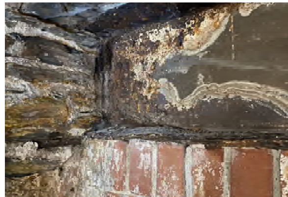
BMR Photo 4.6.B: Heavily corroded steel girder beam at foundation bearing point. Requires immediate attention (1 Mar 2022).
