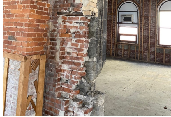
BMR Photo 4.4.B: Damaged load-bearing masonry below west end of steel header beam at 1947 addition opening (28 Feb 2022).
