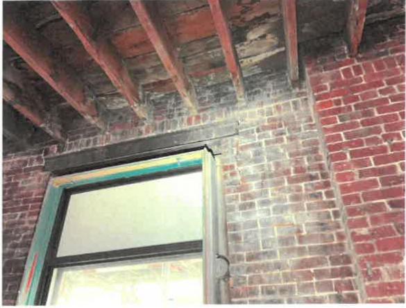
Photo No. 20 – Steel lintel over window with jamb brick cracking at window head. Note water staining of wood framing above.
