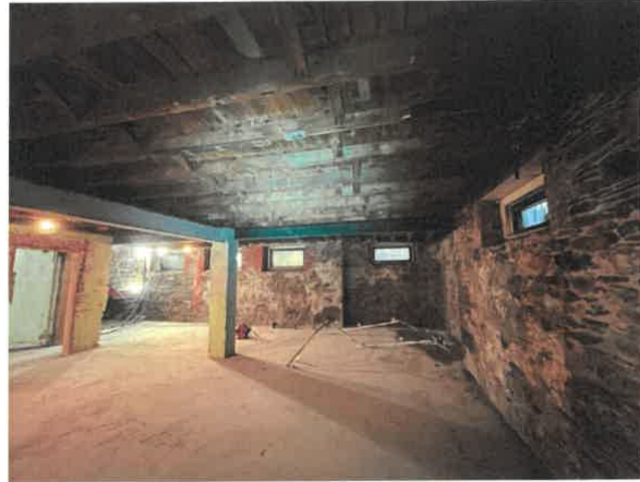
Photo No. 10 – View of 1914 basement masonry walls and wood framing overhead. Interior support girders and concrete encased columns visible.
