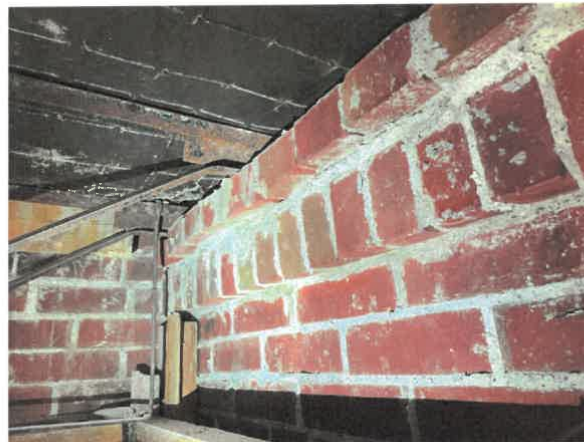
Photo No. 16 – Limited OWSJ bearing on brick corbel at exterior load bearing masonry wall – 1947 addition.
