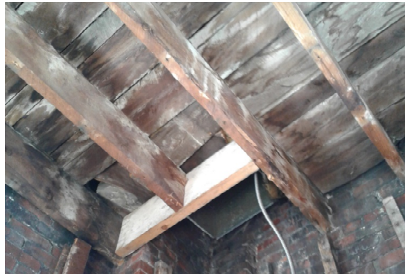
BMR Photo 4.2.B: Water stained/damaged roof joists bearing on masonry wall (28 Feb 2022).
