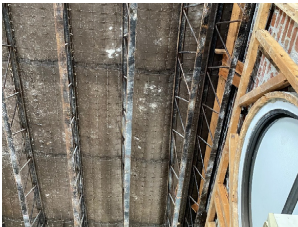
BMR Photo 4.4.E: Failed roof joists at 1947 addition shown buckled out of plane. No bracing or bridging present (28 Feb 2022).
