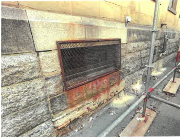
Photo No. 8 – Deteriorated joints and below sill infill at foundation wall opening.
