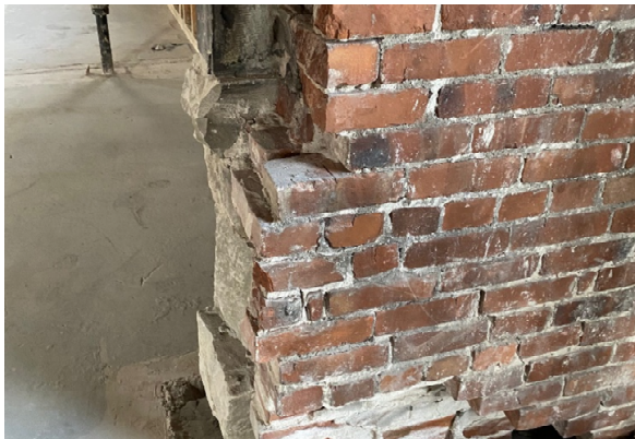
BMR Photo 4.4.C: Damaged and loose load-bearing masonry below east end of steel header beam at 1947 addition opening (28 Feb 2022).
