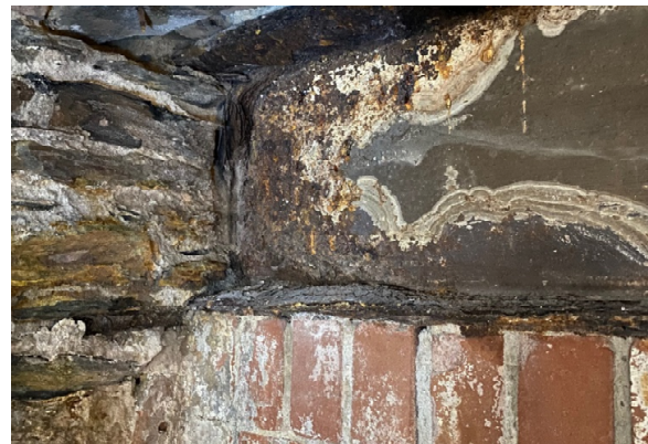
BMR Photo 4.6.B: Heavily corroded steel girder beam at foundation bearing point. Requires immediate attention (1 Mar 2022).
