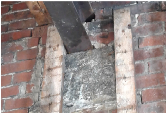
BMR Photo 4.2.C: Granite bearing block at steel girder beam within load-bearing masonry wall. Degraded mortar joints present in masonry walls (28 Feb 2022).
