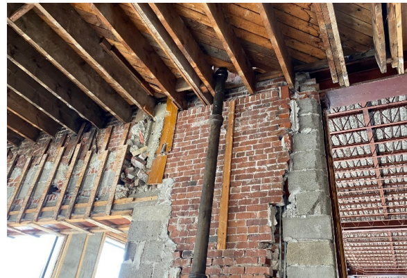
BMR Photo 4.4.D: Loose and damaged load-bearing masonry above and adjacent header beams into 1961 addition (28 Feb 2022).
