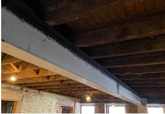
BMR Photo 4.6.E: Steel girder beam, 2"x12" joists, 3"x12" joists all require reinforcement (1 Mar 2022).
