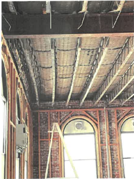
Photo No. 15 – Curved and out of plumb open web steel joists (OWSJ) in roof of 1947 addition.
