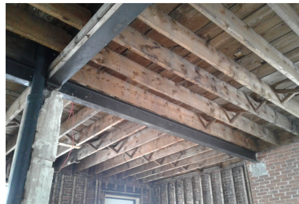
BMR Photo 4.2.D: 2"x10" timber joists supported on steel girder beams and concrete-encased W-columns (28 Feb 2022).
