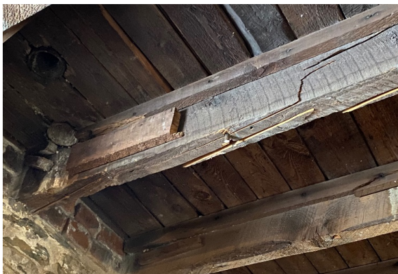
BMR Photo 4.6.C: Timber floor joist that appears to have failed at the bearing point (1 Mar 2022).
