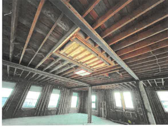
Photo No. 18 – Interior grid steel girders supporting roof. Note wood headers at former roof opening.
