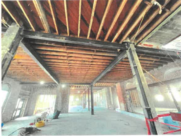
Photo No. 13 – 1914 Main level view looking through openings in 1914 west and north walls with 1961 addition beyond and 1947 addition to the right.
