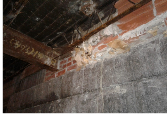
BMR Photo 4.6.F: Corroded steel floor joists and steel girder beam at 1947 addition. Recommend floor be demolished and replaced (1 Mar 2022).
