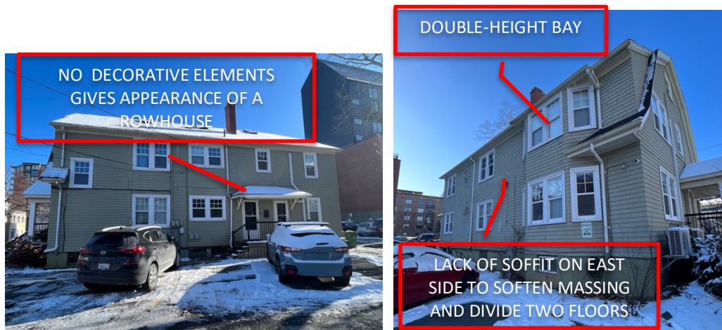
Figure 35b: Side components of 43-45 Dundas Street that detract from the style and overall design of a Dutch Colonial Revival house.
