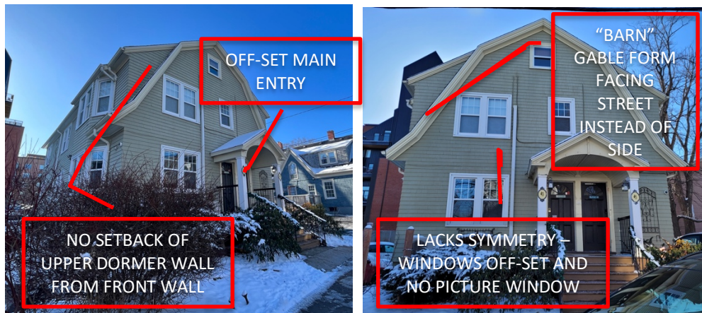
Figure 35a: Front components of 43-45 Dundas Street that detract from the style and overall design of a Dutch Colonial Revival house.
