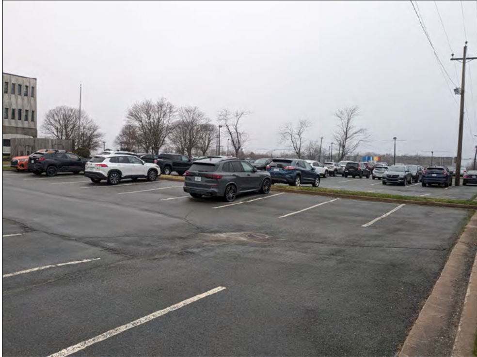
Plate 12: Wastewater drain in parking lot at the north of the Research Drive complex with linear cracks, looking west. In background note power poles and streetlights without overhead powerlines.
