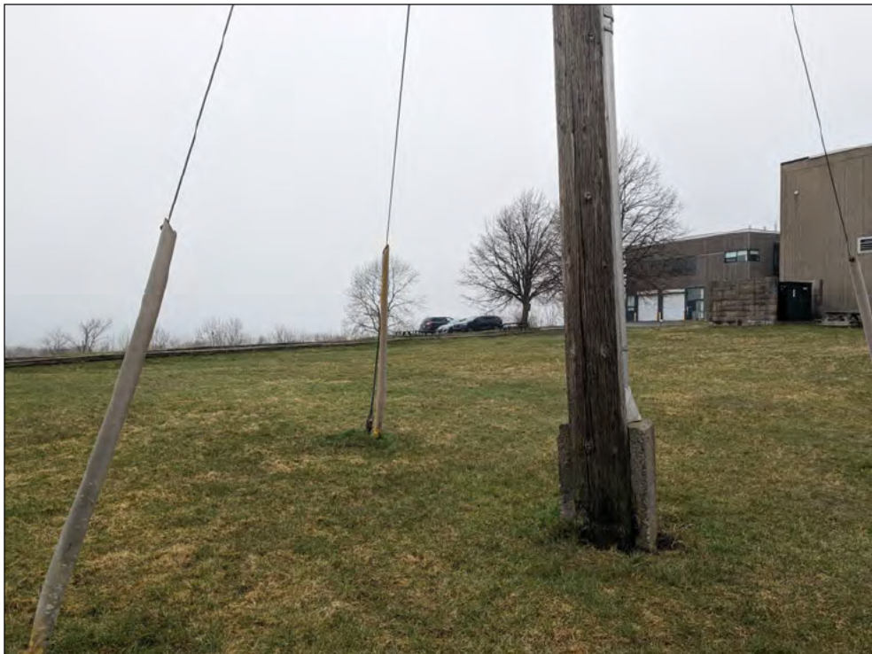
Plate 13: Electrical conduit on the east of the Research Drive buildings, looking west.
