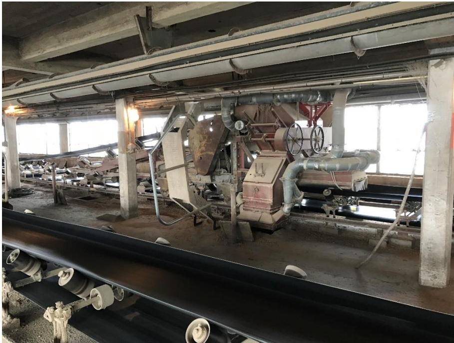
D.18: Belt tripper in Annex 2.
