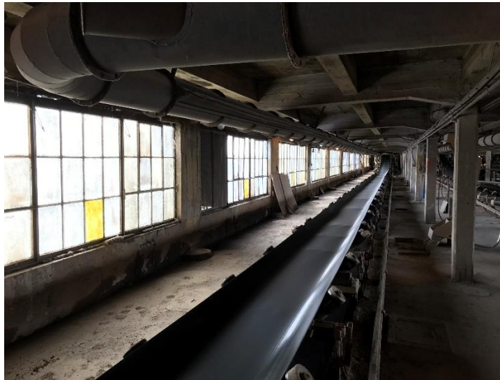
Figure 3.4: Photograph of windows and vent opening along the exterior walls in Annex 1.
