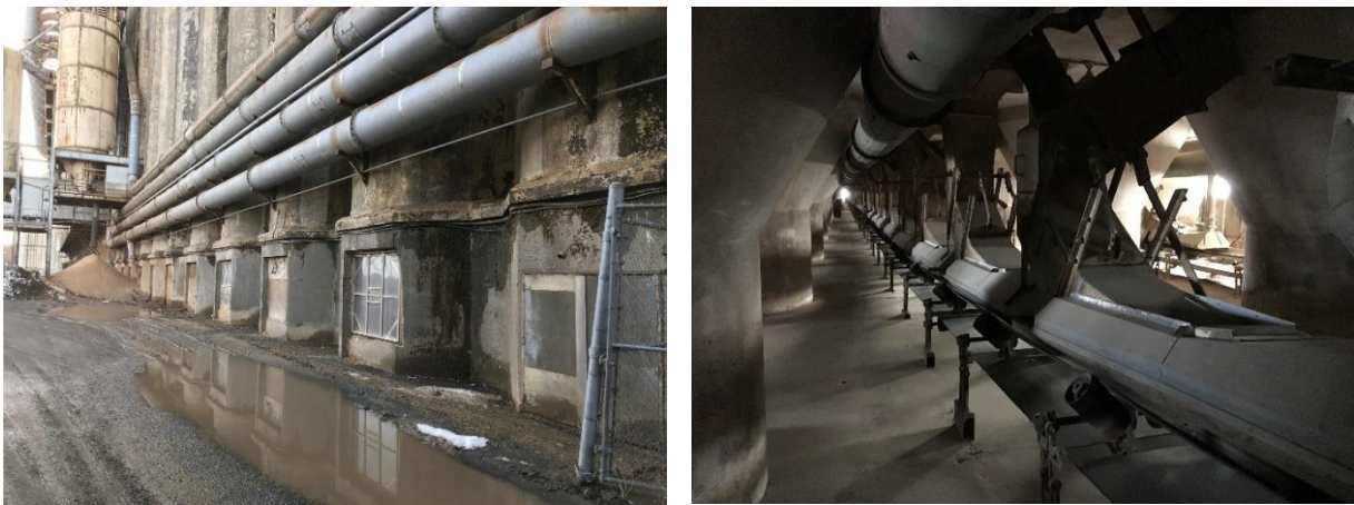
Figure 2.6: Exterior of Annex 1 basement gallery (left) and interior of Annex 3 basement gallery (right).
