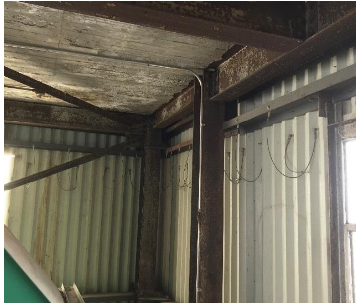
Figure 3.2: Photograph of the explosion release cladding on the exterior walls in Workhouse #3.
