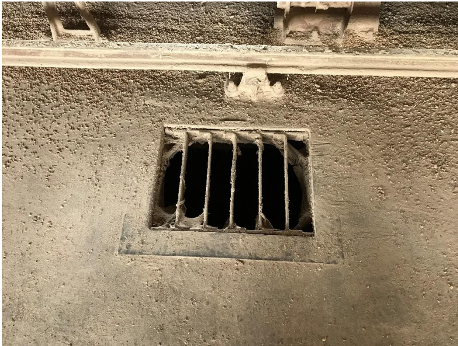
D.14: Silo chute in the Annex 1 bin level gallery.
