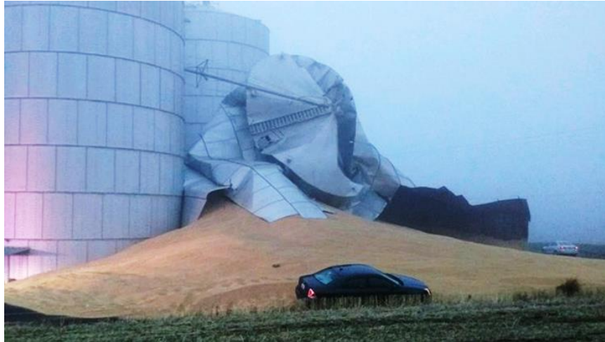
Figure 8.4: Example of bulk material outflow from a ruptured grain silo.
