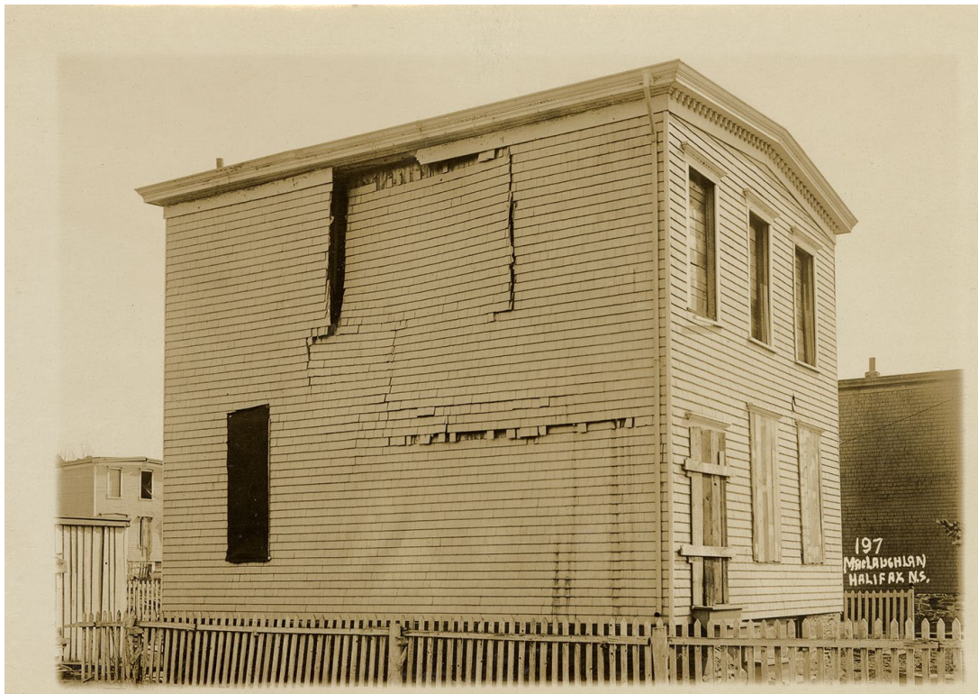
Figure 31: Damaged house on Windmill Road of similar style to 20 Ropewalk Lane (MacLaughlan, Album 2, No 197).
