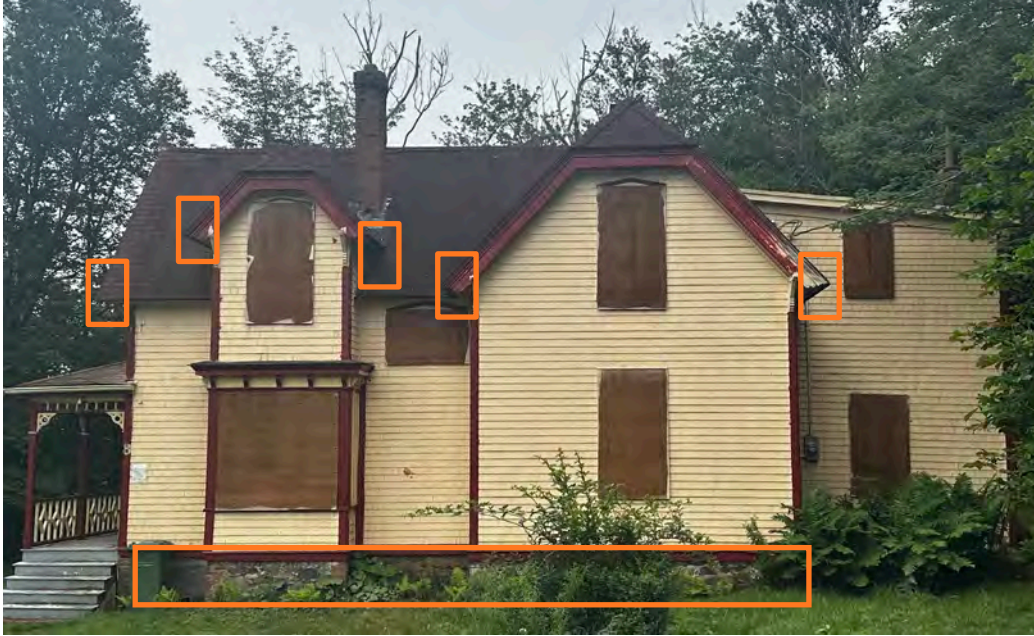
Figure 9: Red Gables north elevation with the foundation outlined in blue and the consistent gable brackets outlined in orange (Staff photo, July 17th, 2024)
