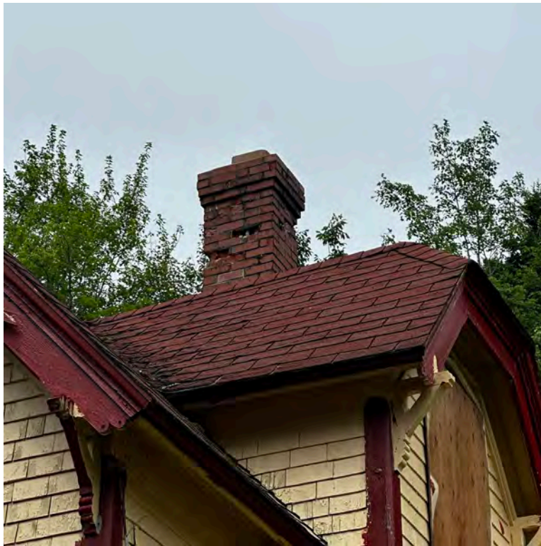
Figure 12: Brick chimney located above the gabled dormer on the north elevation (Staff photo, July 17th, 2024)
