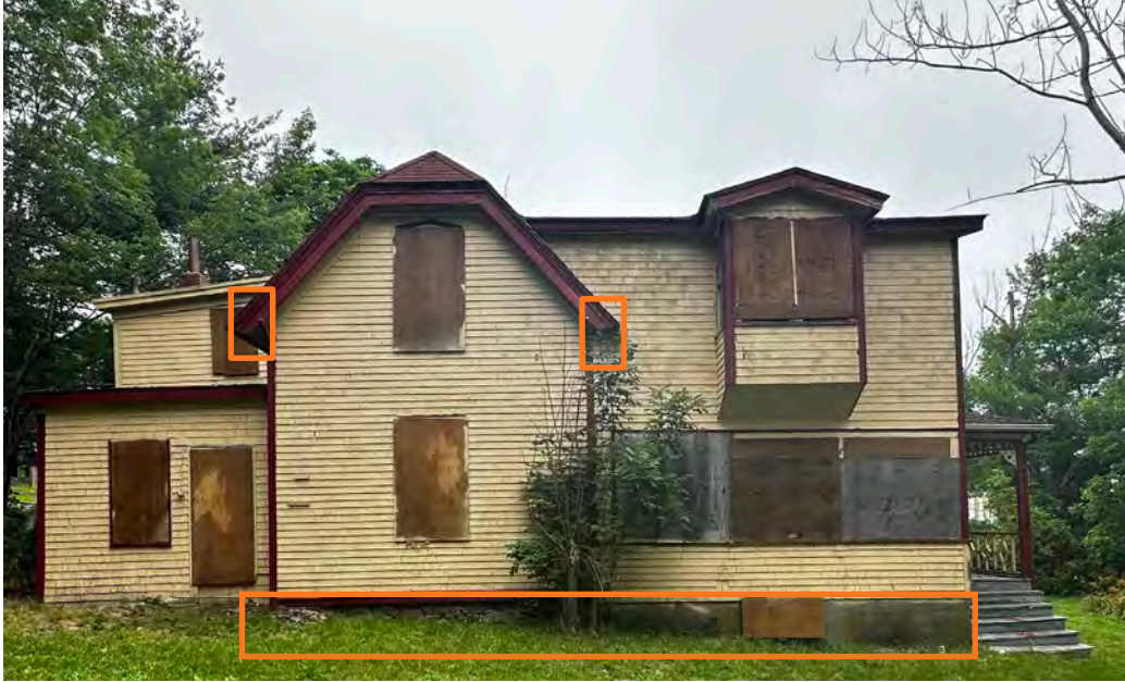
Figure 10: Red Gables from south elevation with the foundation outlined in blue and consistent brackets outlined in orange (Staff photo, July 17th, 2024)
