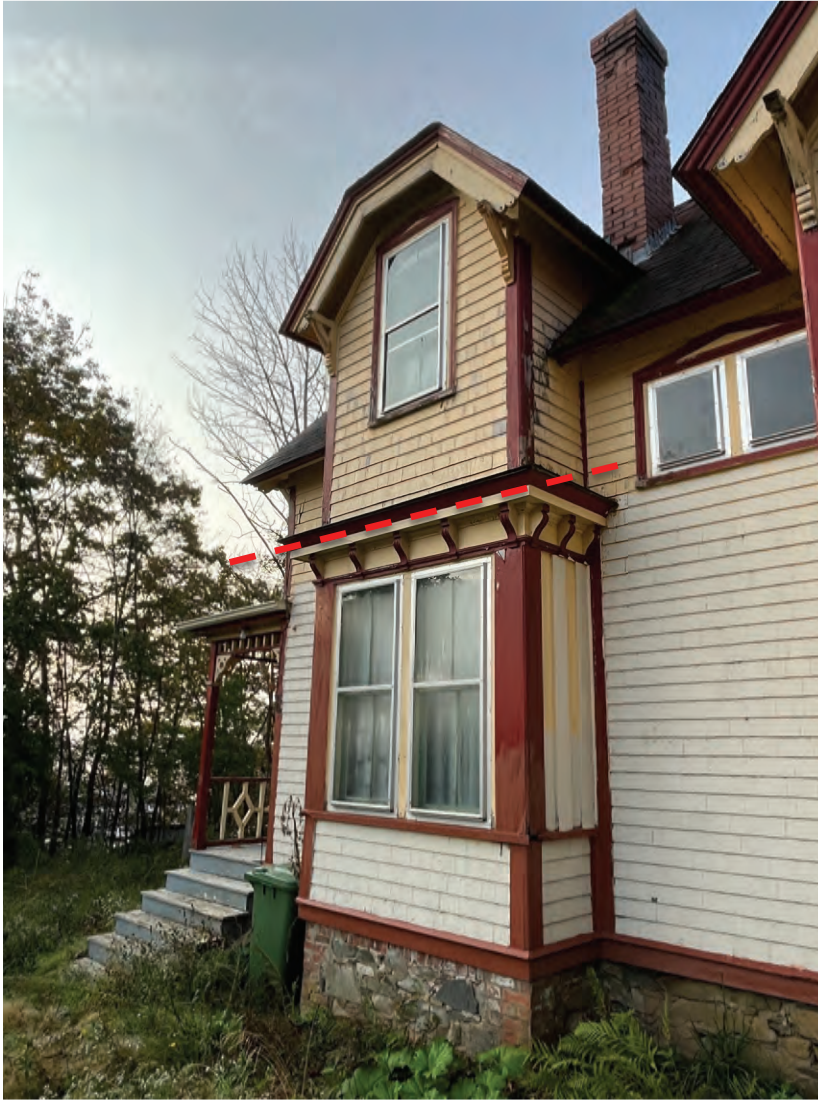
Figure 22: North side bay – original c. 1870 portion below dashed line and 1917 addition above dashed line to create a wall dormer.
