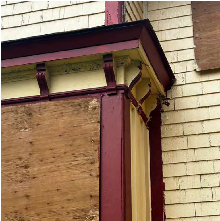
Figure 15: Decorative brackets and siding of the bay window (Staff photo, July 17th, 2024).
