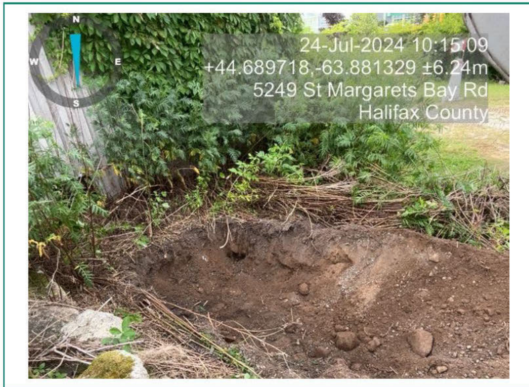
Photo 3: TP1 in location of old, abandoned AST.
