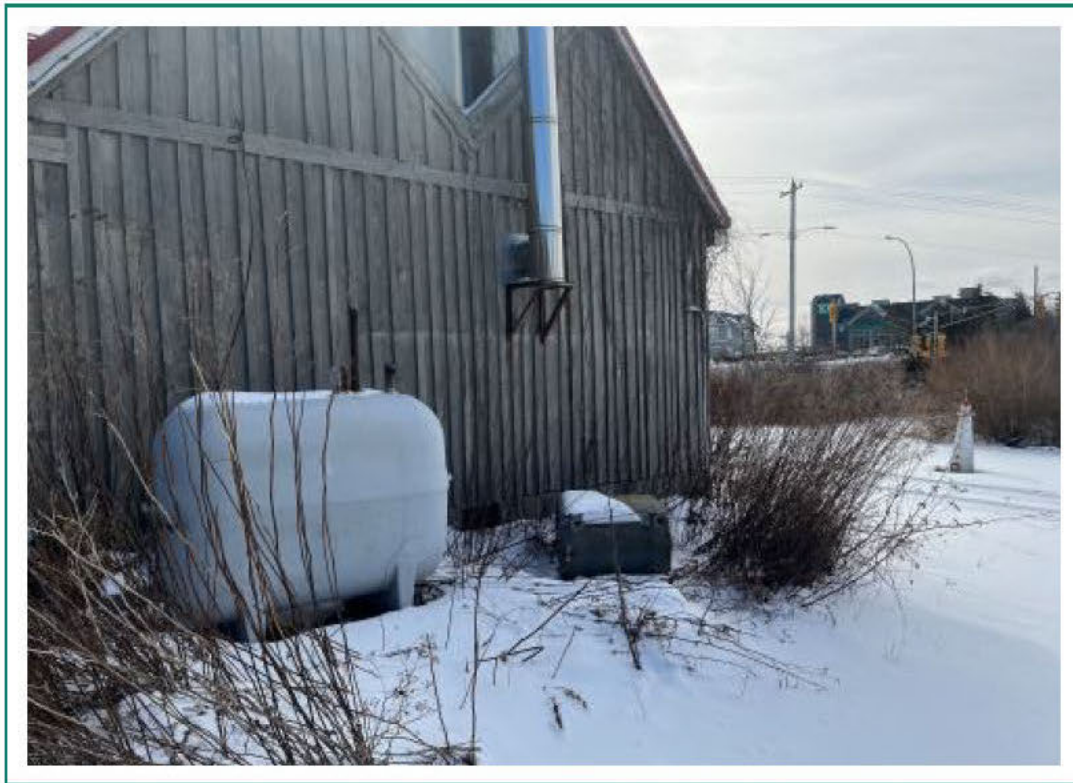
Photo 1: Photo looking south showing fibreglass fuel oil AST and the abandoned steel AST on the west side of 5249 St. Margarets Bay Road (February 28, 2023).
