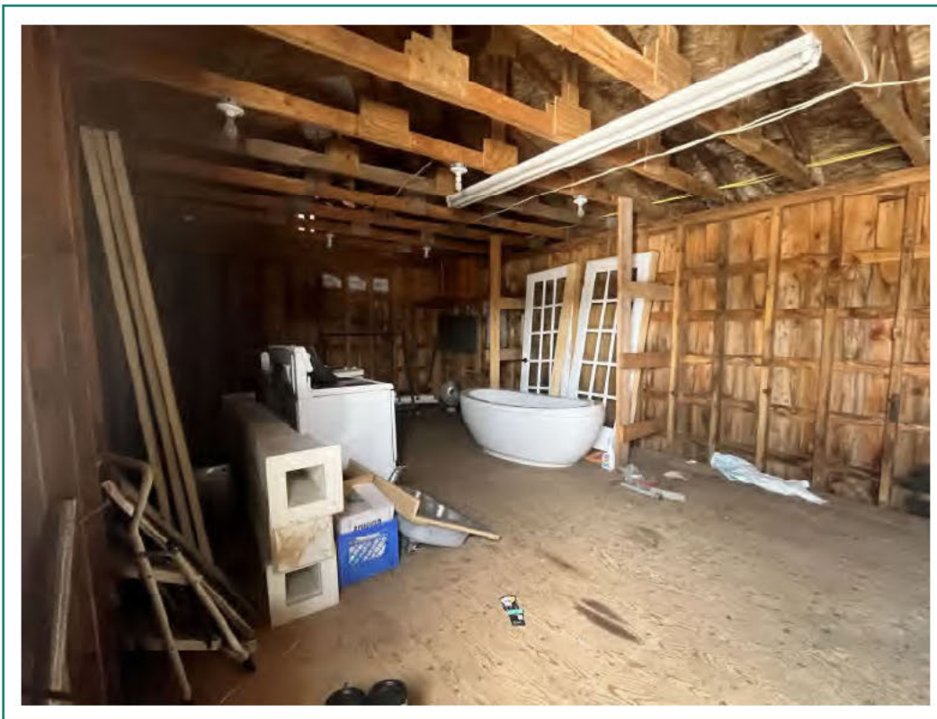
Photo 10: View looking northeast from the doorway of the storage building west of 51 Sonnys Road in Upper Tantallon, NS (taken February 28, 2023). Note the interior finishes.
