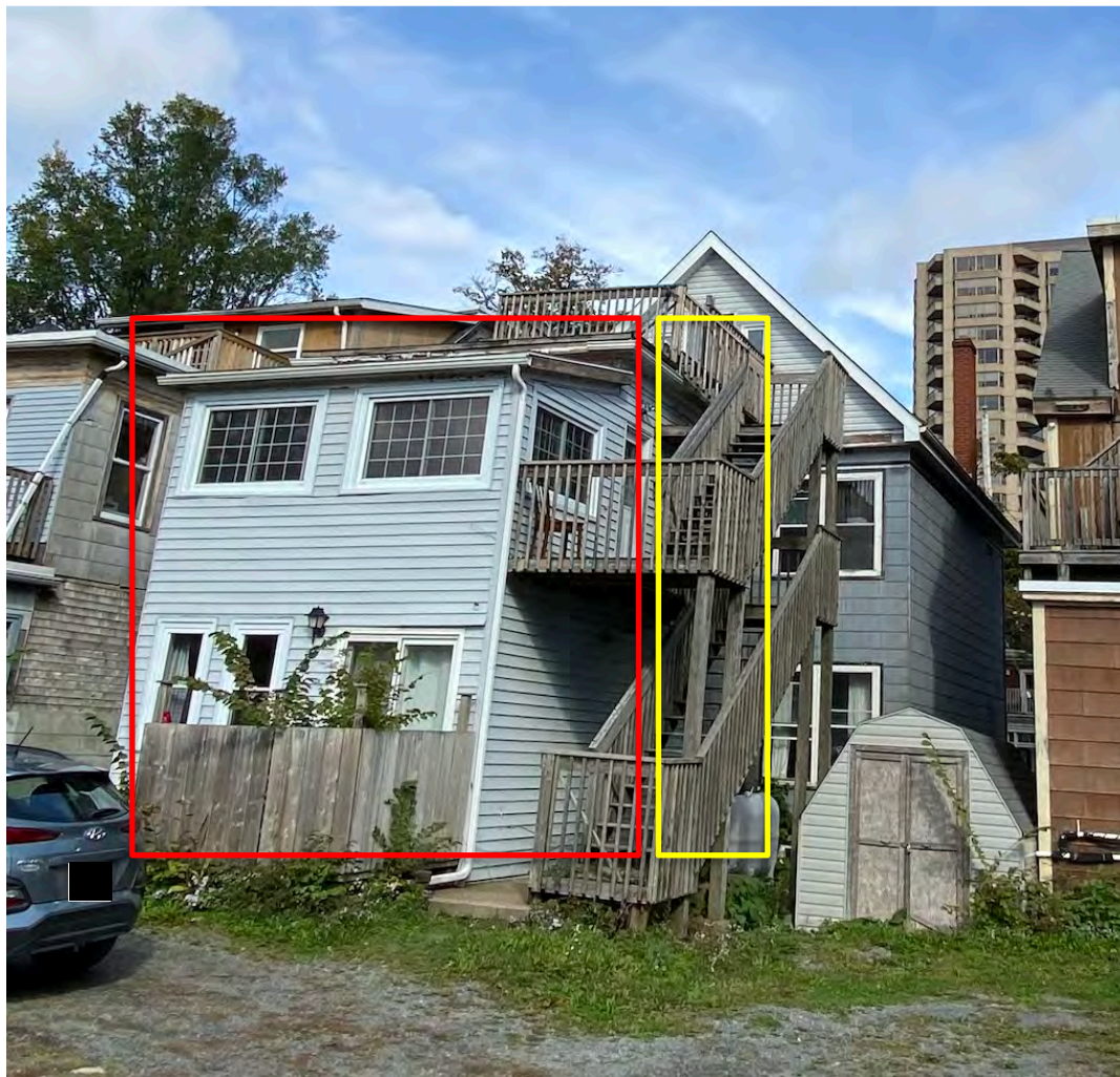
Figure 58: Keith Residence, 1466 Carlton Street – additions to the rear: 1907-1914 (yellow), later date (red)
