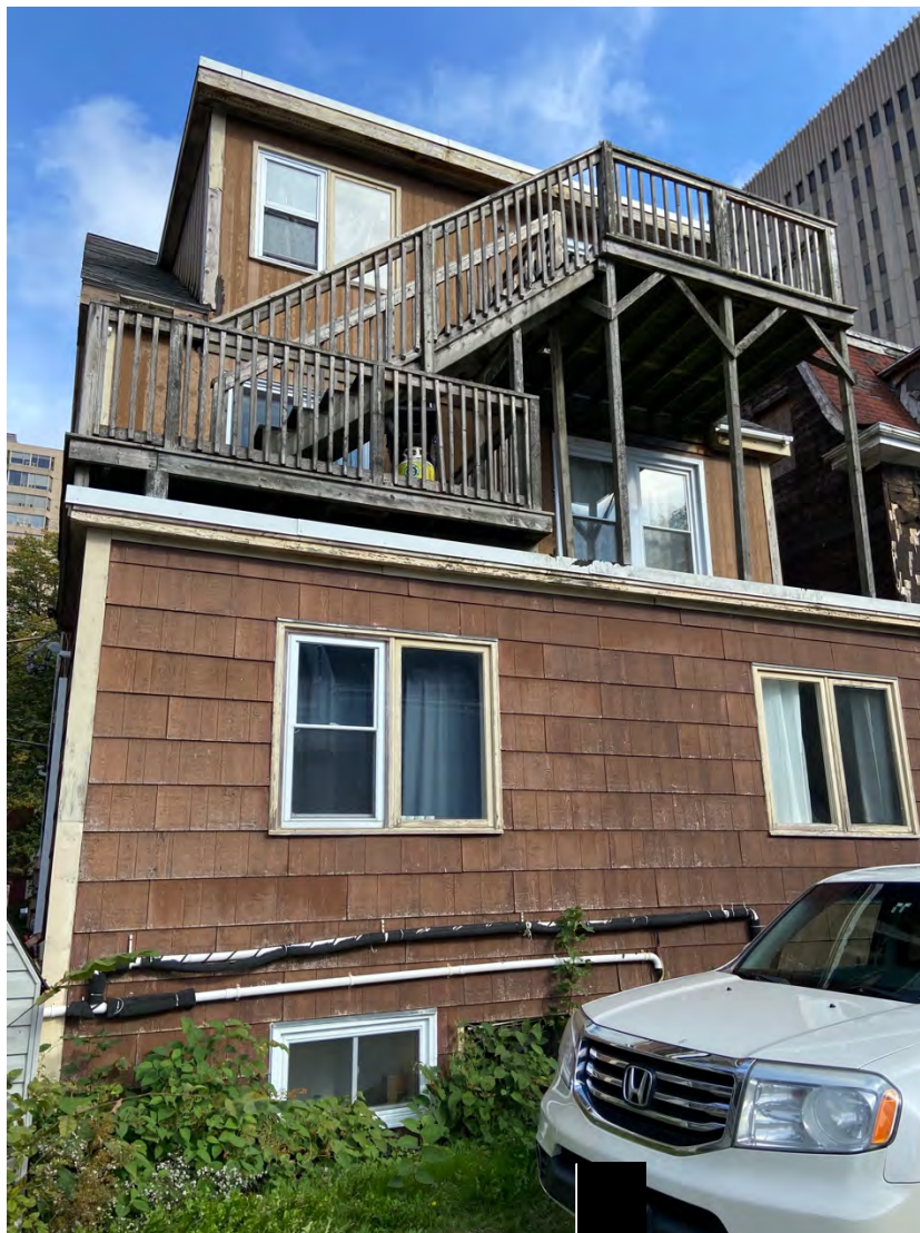
Figure 48: Extension to the main floor and basement, and attic shed dormer with fire escape at the rear of 1460 Carlton Street
