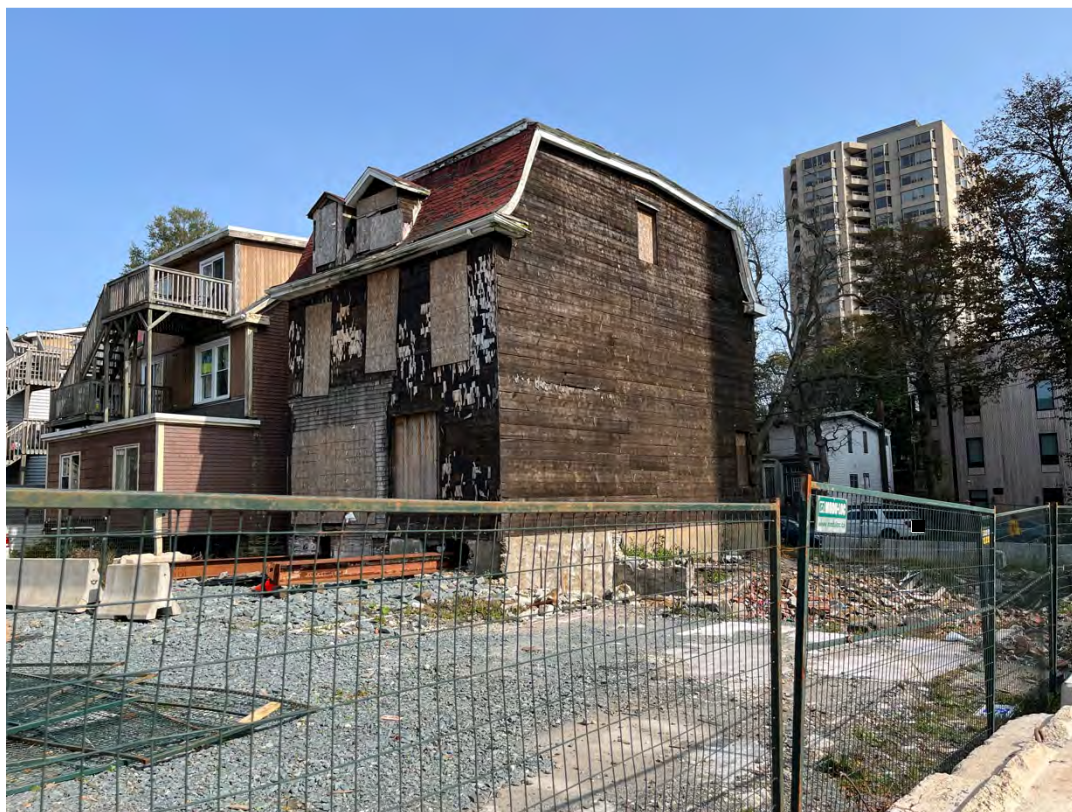
Figure 35: 1456 Carlton Street following unauthorized alterations (rear and south side)
