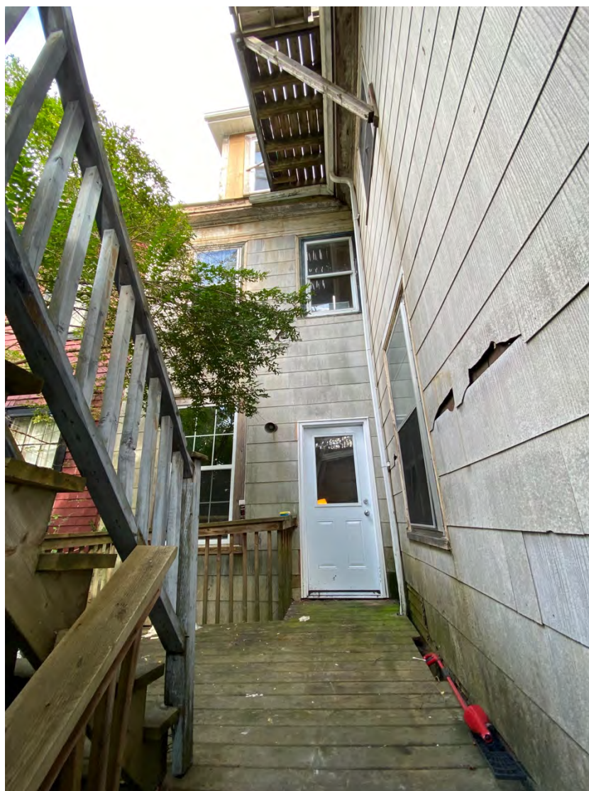
Figure 63c: Tupper Residence, 1468 Carlton Street, inset rear – north half comprising an earlier two-storey extension (c. 1910)
