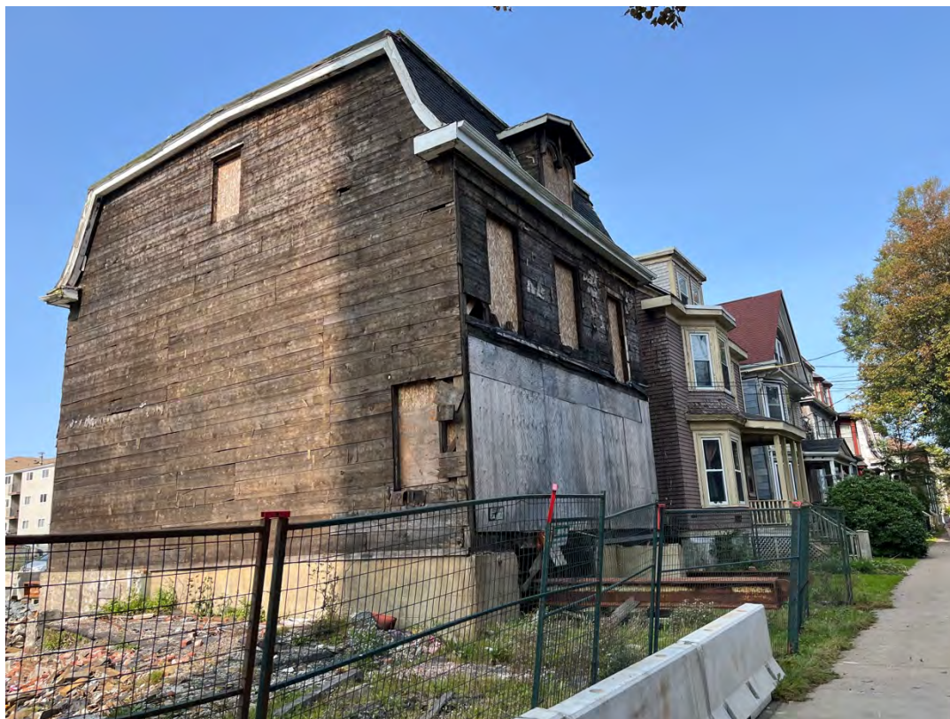
Figure 34: 1456 Carlton Street following unauthorized alterations (front and south side)
