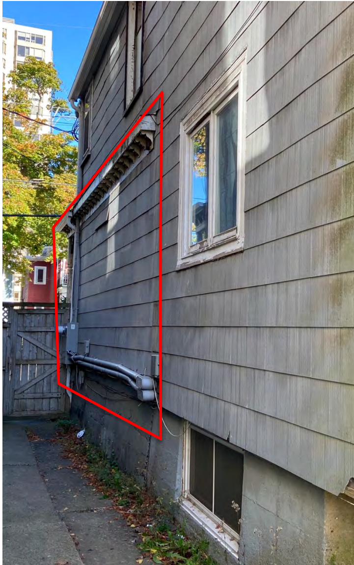
Figure 56: Remnants of wrap-around porch (roof line and brackets), and full extent of that side of porch outlined, north side
