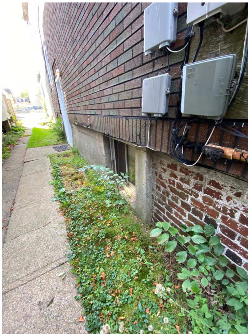
Figure 72e: Tupper Residence, 1468 Carlton Street – south side foundation comprising brick and concrete
