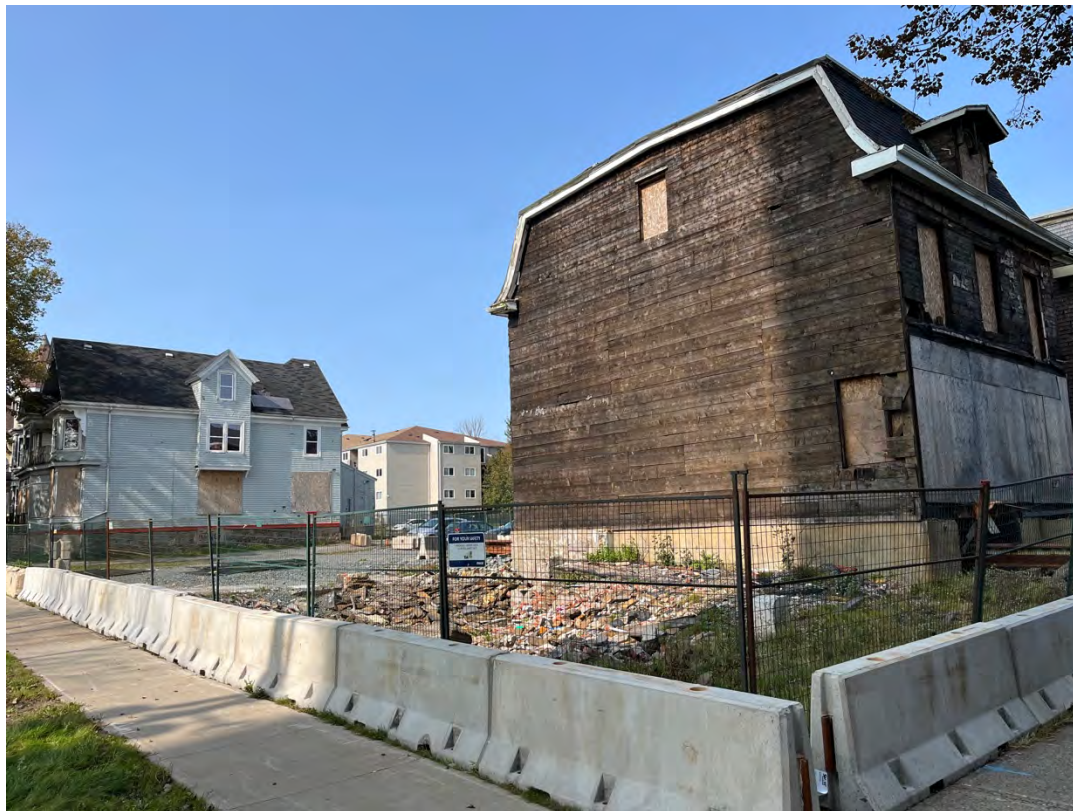
Figure 33: Corner of Carlton and College Street – vacant site following the collapse of the house previously located here
