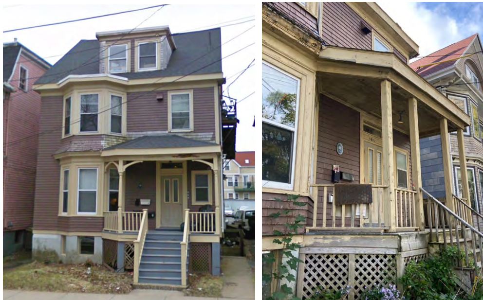
Figure 45: Front porch details of 1460 Carlton Street, April 2009 (left) and October 2024 (right)
