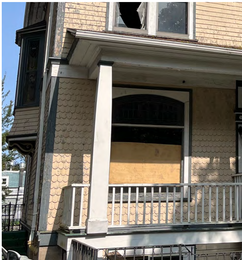
Figure 29: Gold Cure Institute, 5969 College Street – front porch and fixed front window with arched top sash
