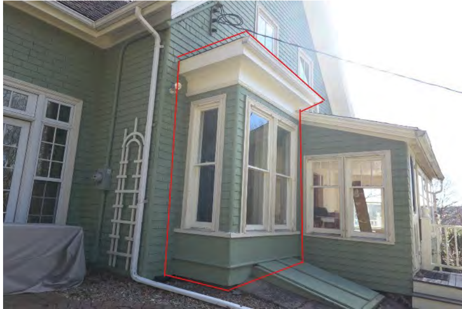
Figure 20: Box bay window adjacent to the south addition, with a hipped roof, cornice trim, and wood windows, recognized as a character-defining element (Staff photo, April 18, 2024)
