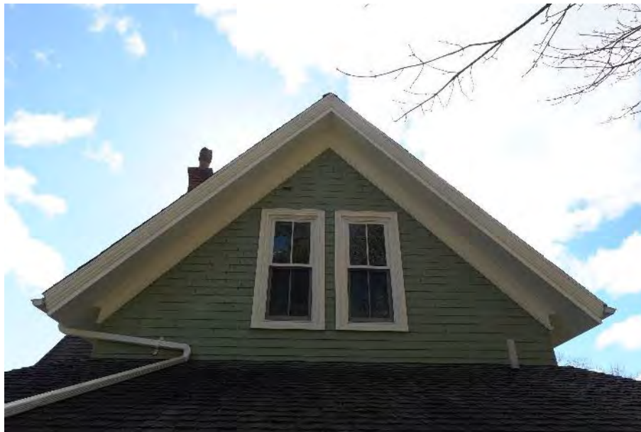
Figure 16: Fascia boards and frieze trims and two tall narrow wood windows on the rear gable (Staff photo, April 18, 2024)
