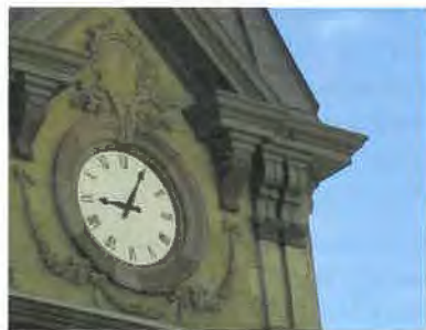
North Clock face permanently fixed to 9:04.35
