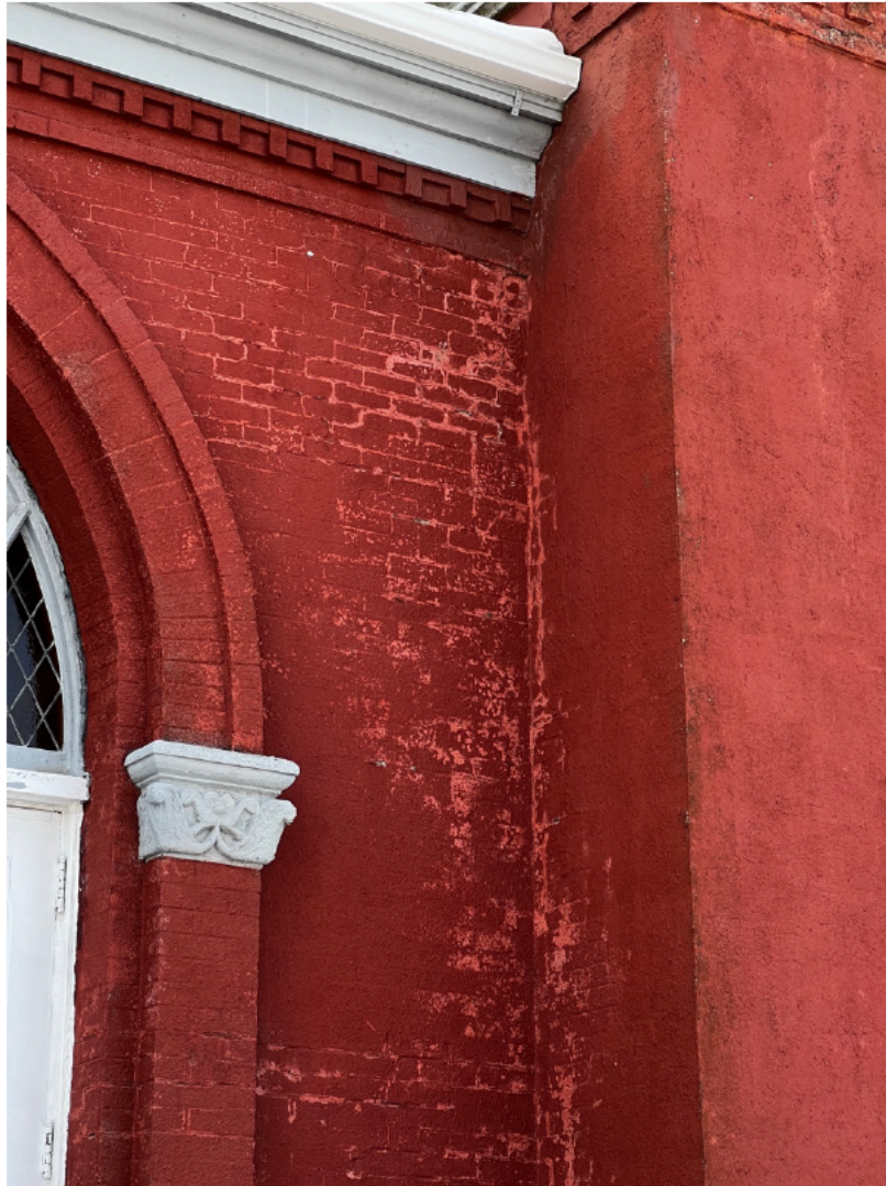
Figure 41e: St. Mark's Church, 5522 Russell Street (connection between entry wall and north tower)
