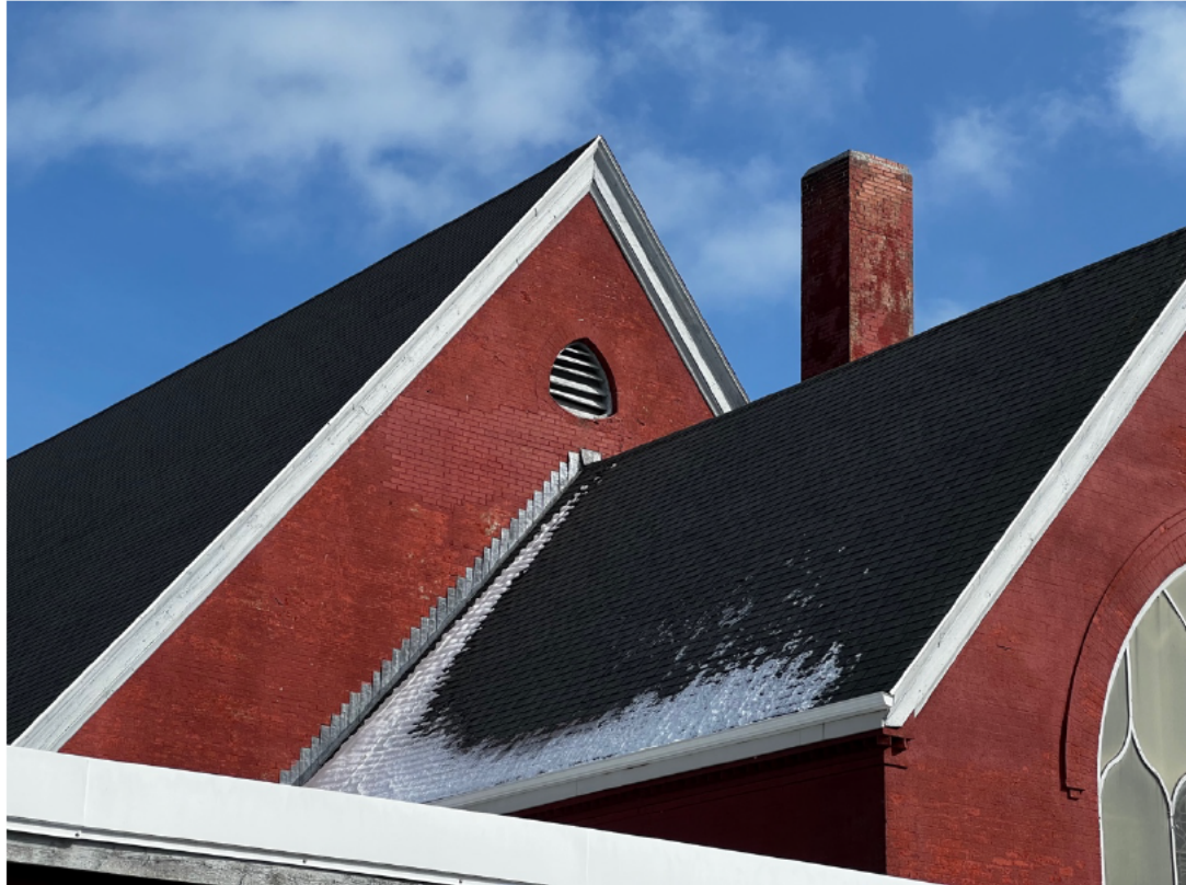
Figure 41m: St. Mark's Church, 5522 Russell Street (rear walls of main body and apse)
