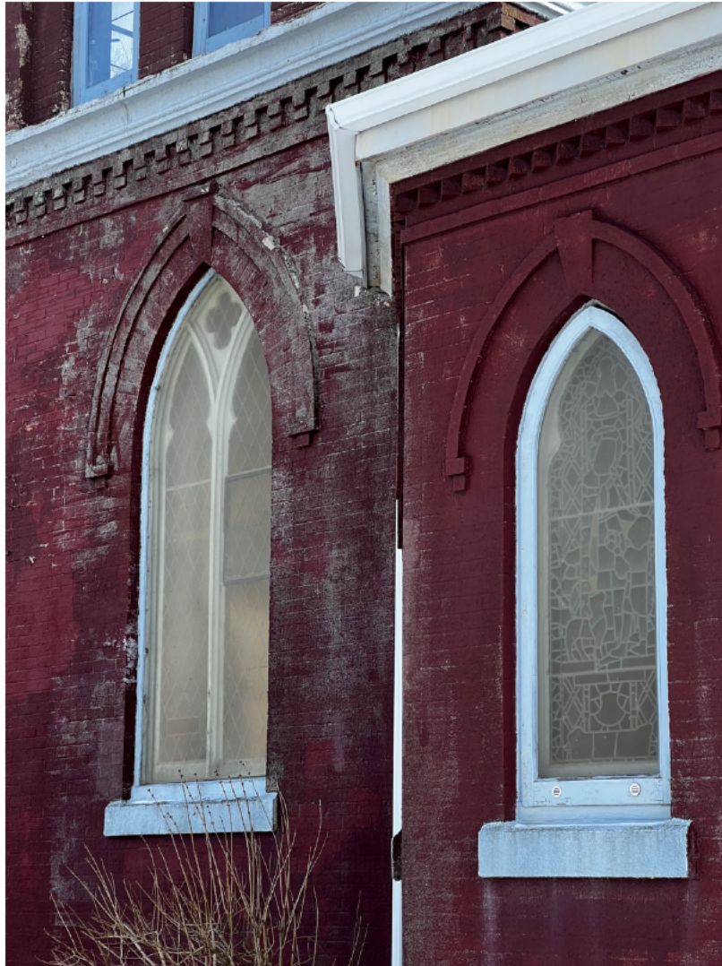
Figure 41k: St. Mark's Church, 5522 Russell Street (connection between base of north tower and protruding alcove)
