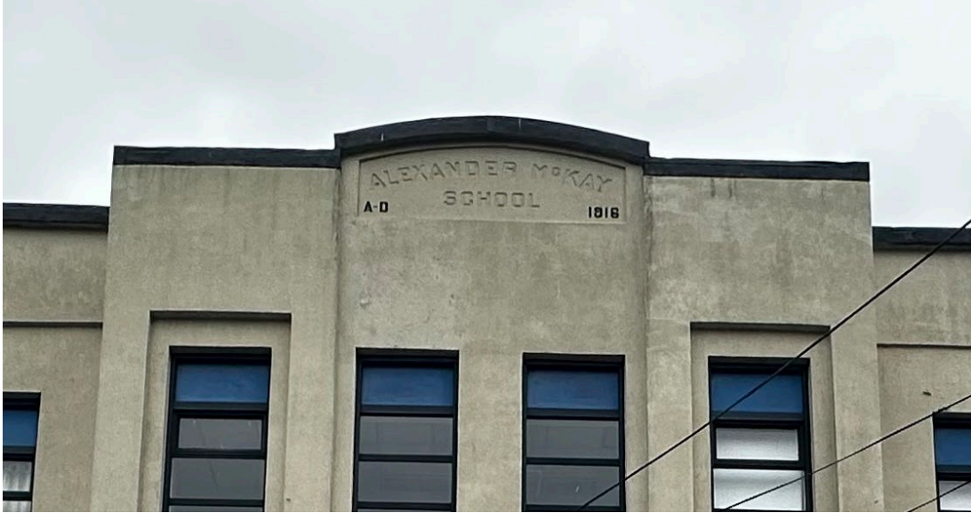
Figure 19: Inscription Stone as visible from the north elevation of original building (May 1, 2024)
