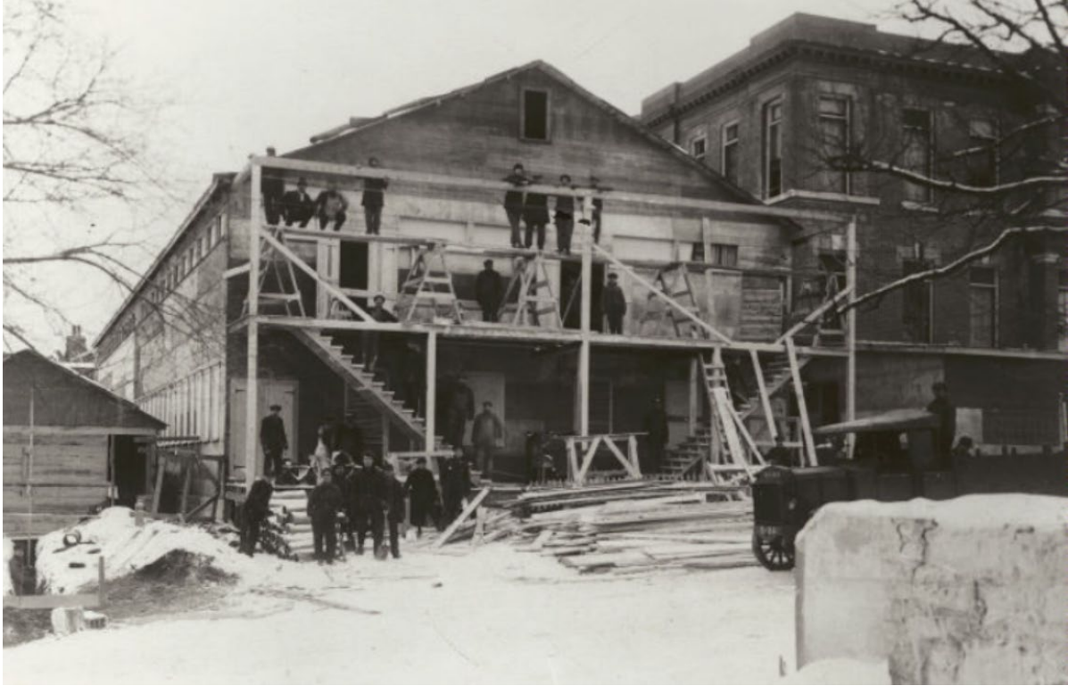
Figure 3: Temporary Dining Hall for Reconstruction Workers behind Alexander McKay School, 1918 (Source: Nova Scotia Archives)
