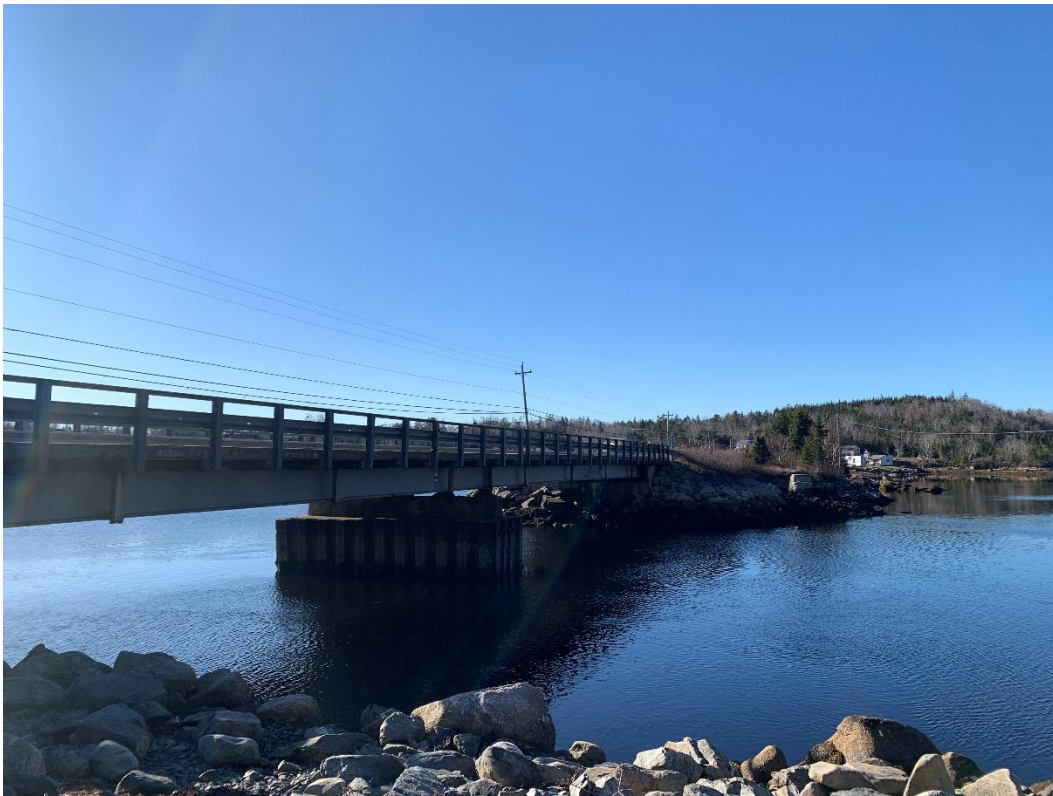
Figure 11-11: The Salmon River Bridge deployment site.
