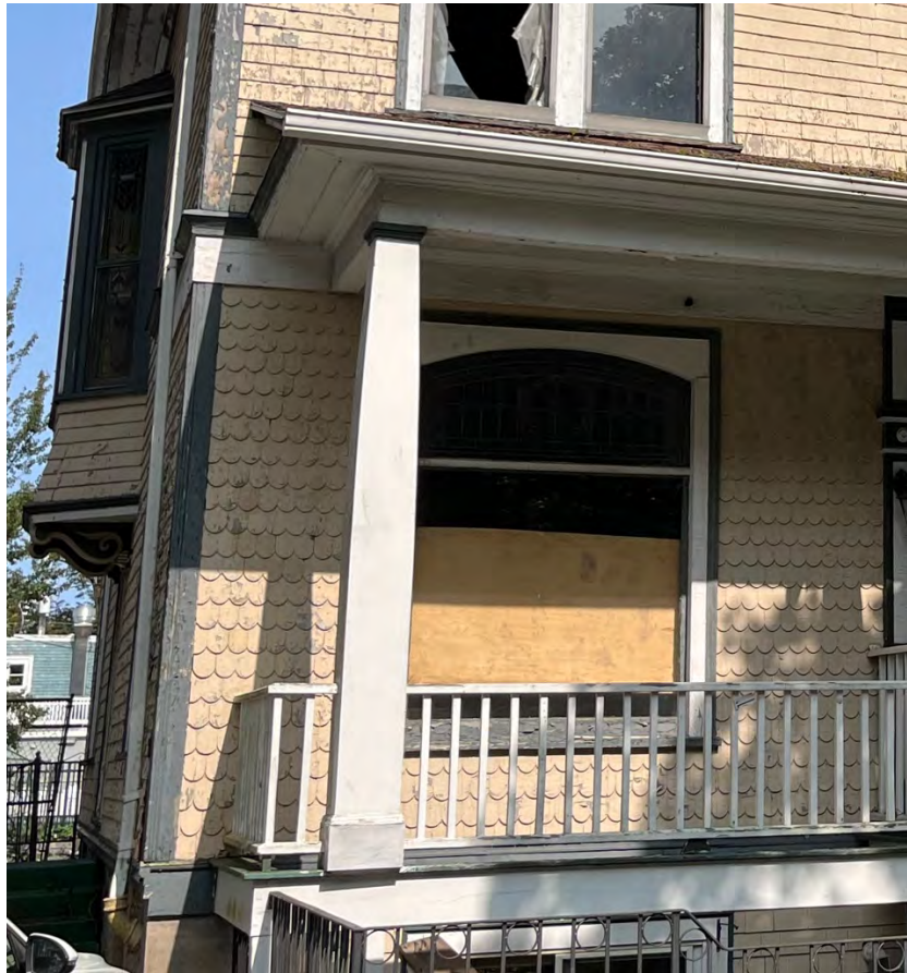
Figure 28: Gold Cure Institute, 5969 College Street – front porch and fixed front window with arched top sash
