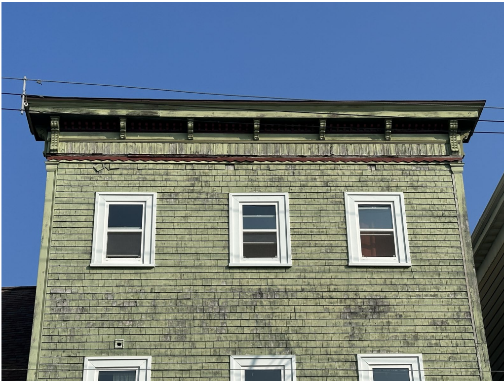
Figure 13: Decorative bracketed cornice and corner boards on the south elevation of 5561 Cogswell Street. The prominent cornice, brackets and decorative trim is the work of the late Hal Forbes (September 2023)
