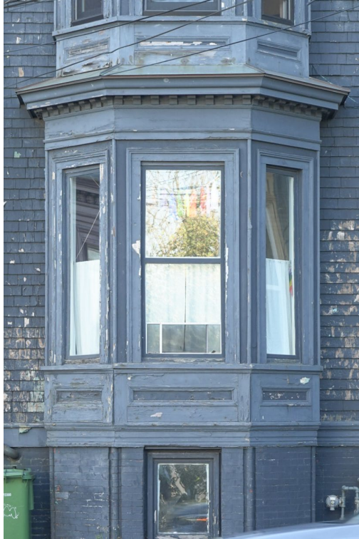
Figure 14: Details of front bay window (October 23, 2023)
