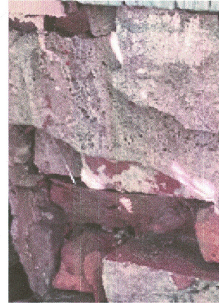
Fig. 35 Foundation structurally unsound, stones/brick falling apart will be replaced with antique style bricks
