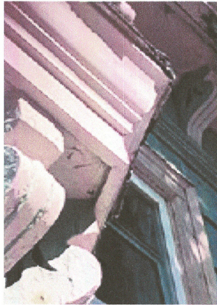
Fig. 33 Wood work will be scraped and repainted if not rotten or replaced using the original patterns.
