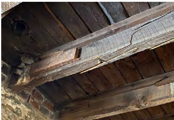
BMR Photo 4.6.C: Timber floor joist that appears to have failed at the bearing point (1 Mar 2022).
