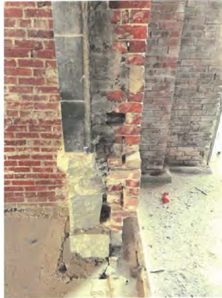
Photo No. 14 – Opening through existing wall with window sill cut out. Sandstone facing with three wythe brick back up wall.
