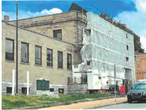
Photo No. 1 – View from Queen Street – South Elevation. Low roof area at left side will be demolished.
