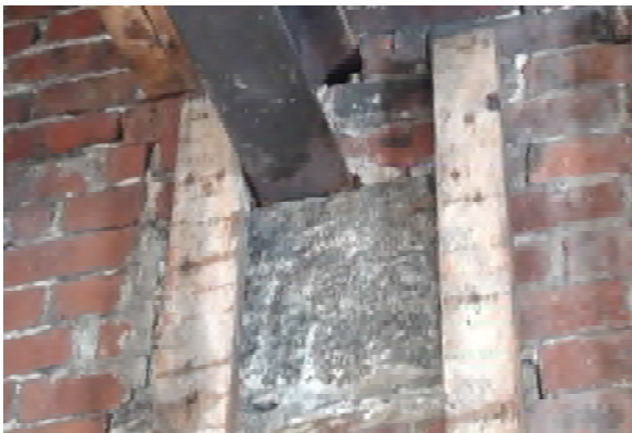
BMR Photo 4.2.C: Granite bearing block at steel girder beam within load-bearing masonry wall. Degraded mortar joints present in masonry walls (28 Feb 2022).
