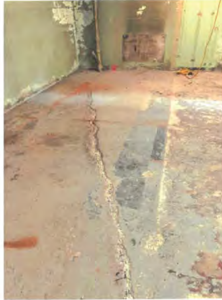
Photo No. 26 – Slab on grade crack in floor – 1947.
