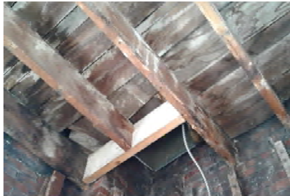
BMR Photo 4.2.B: Water stained/damaged roof joists bearing on masonry wall (28 Feb 2022).
