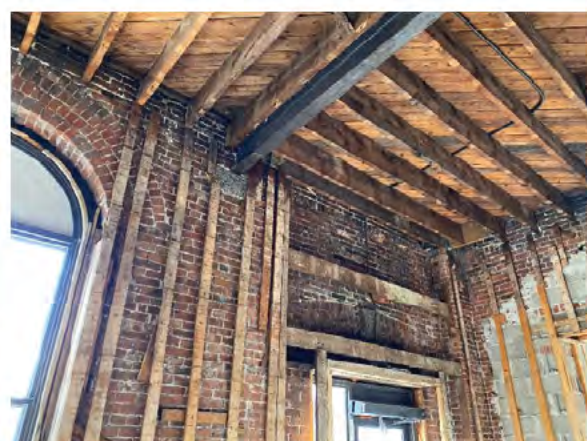
BMR Photo 4.4.F: Timber joists bearing on exterior masonry wall. Girder beam bearing on granite block (28 Feb 2022).
