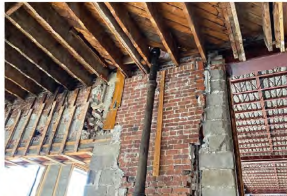
BMR Photo 4.4.D: Loose and damaged load-bearing masonry above and adjacent header beams into 1961 addition (28 Feb 2022).
