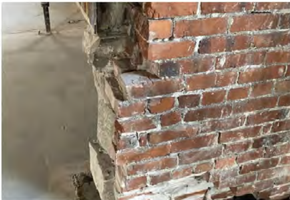
BMR Photo 4.4.C: Damaged and loose load-bearing masonry below east end of steel header beam at 1947 addition opening (28 Feb 2022).
