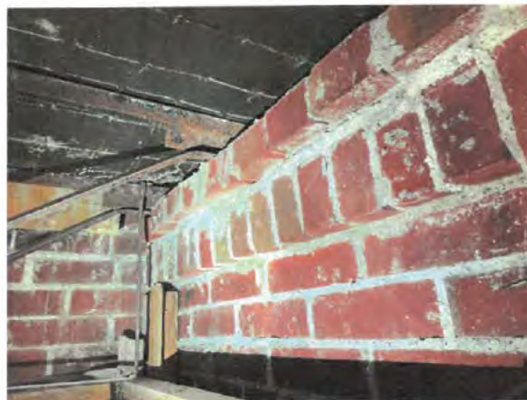
Photo No. 16 – Limited OWSJ bearing on brick corbel at exterior load bearing masonry wall – 1947 addition.
