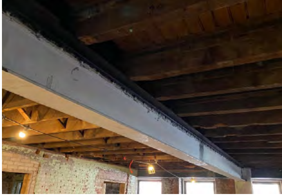
BMR Photo 4.6.E: Steel girder beam, 2"x12" joists, 3"x12" joists all require reinforcement (1 Mar 2022).
