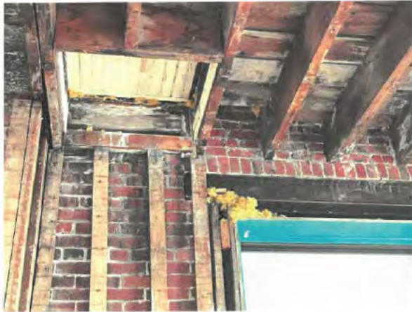
Photo No. 21 – Attic roof hatch at former Clock Tower location (South East).
