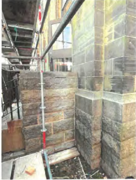
Photo No. 9 – Open joints in granite at east entry area.
