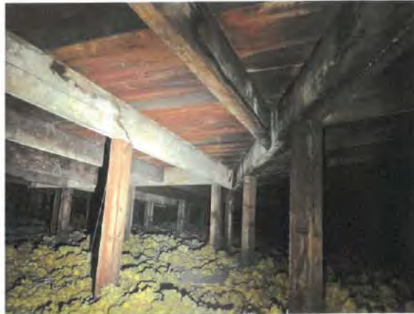
Photo No. 22 – View of attic space. Sloped roof support framing with props to ceiling joists below. Insulation on top of ceiling visible.
