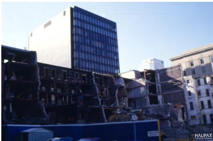
Above: An HRM Archives photo erroneously dated 1987 (likely to be c.1985) showing the rear of the historic facades which were retained as part of the Founder’s Square development.
