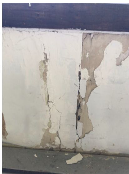
Water damaged drywall underneath sliding window
