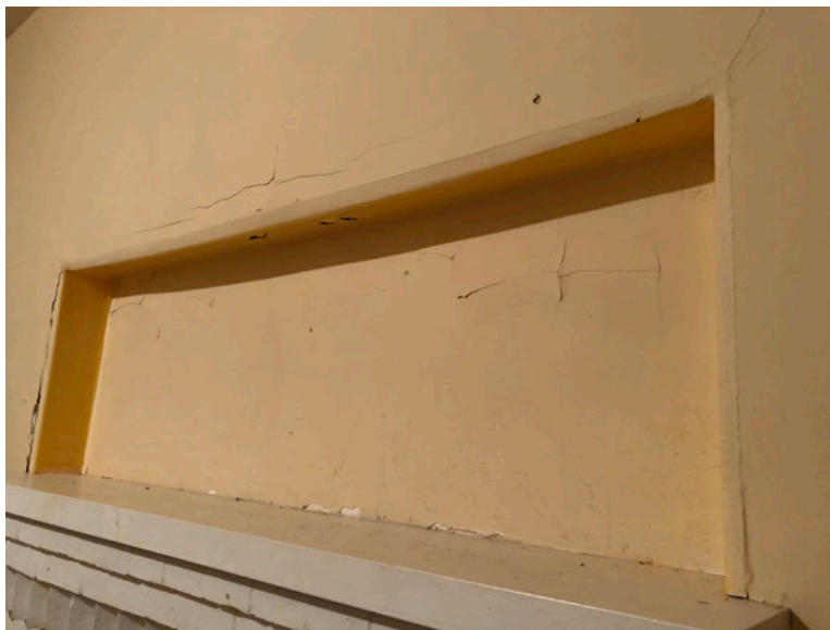
Bowing lintel in kitchen, with cracking plaster or drywall
