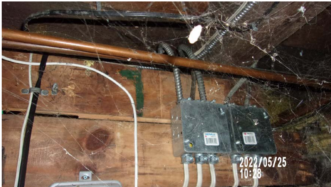
E5- Typical Wiring Methods Observed.
