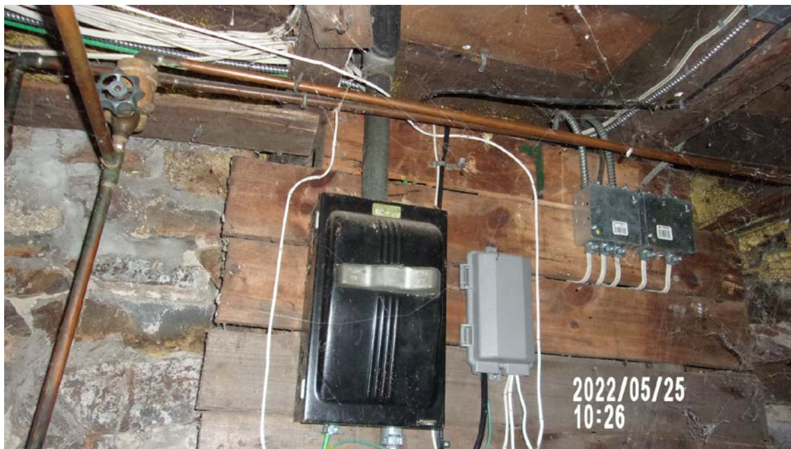
E3- Amalgamated Main Fusible Disconnect Switch Fused at 60 Amps.
