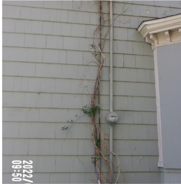
E1-Electrical Mast and Meter Base
