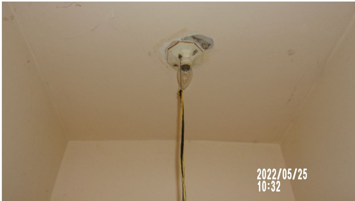
E8- Typical Light Fixture
