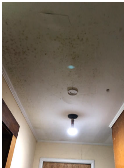
Potential mould in the back hall ceiling
