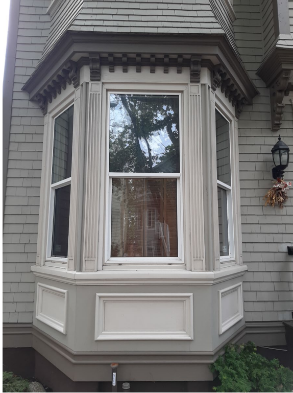
Figure 13: Two-storey Bay window with paneling, wood piers and bracket and corbel detailing on the north elevation (Staff photo, 16 June 2023)
