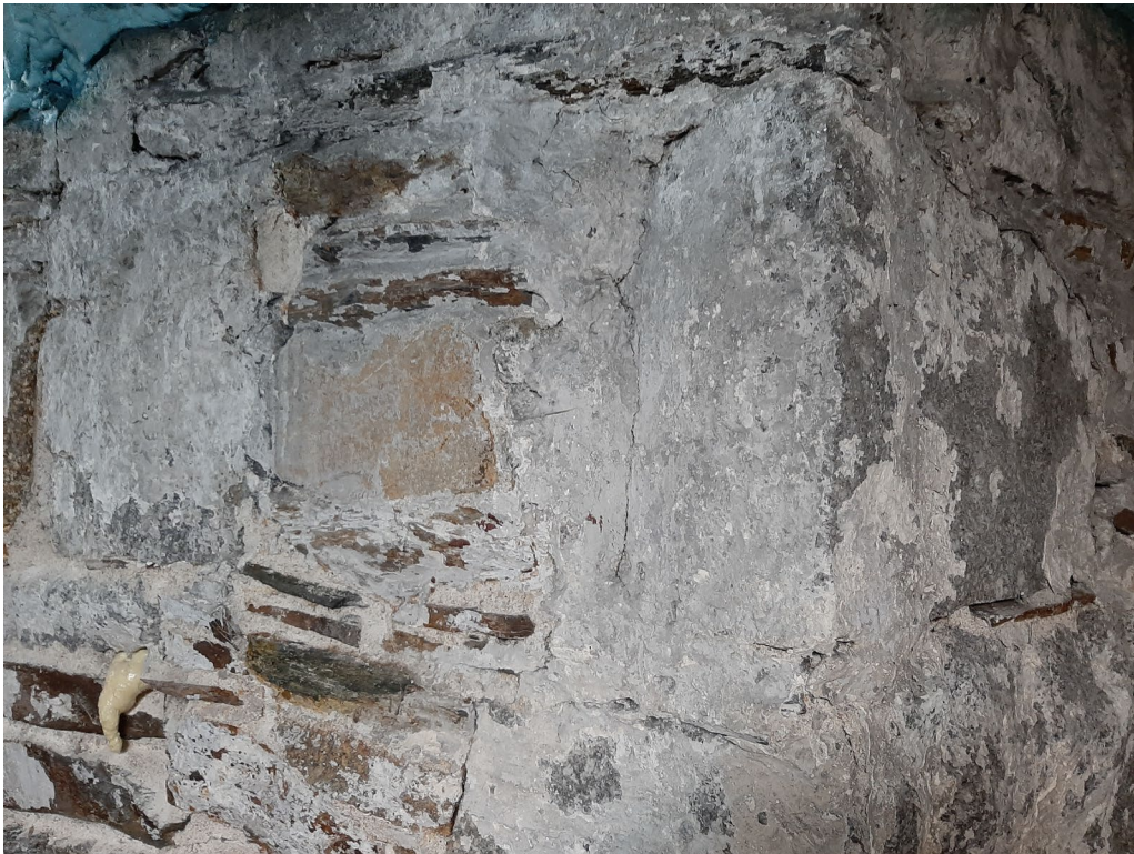
Figure 6: Interior of the foundation as visible from the basement (Staff photo, 16 June 2023)
