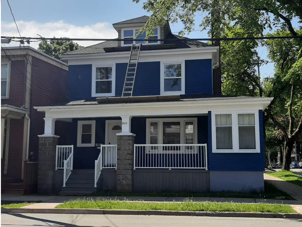
Figure 14: Concrete block veranda posts at 6072 Jubilee Road (Staff Photo, June 16, 2023)
