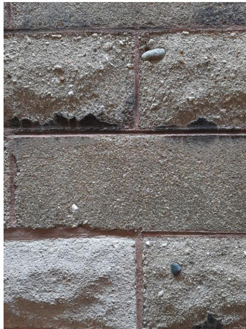
Figure 20: Concrete block cladding of 1741-1743 Henry Street. Note pieces of shell and aggregate incorporated into some of the blocks (Staff Photo, 19 May 2023)
