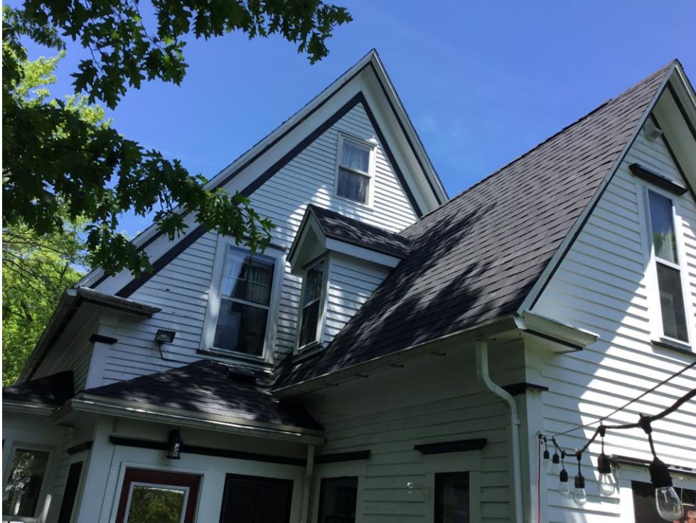
An example property (46 Dahlia St, Dartmouth) whose re-roofing was assisted by the Heritage Incentives Program
