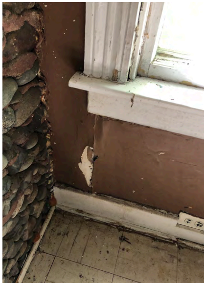
Decaying drywall adjacent to amethyst fireplace in living room
