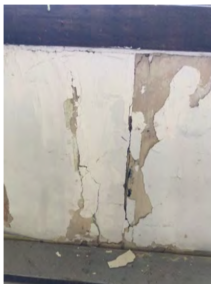
Water damaged drywall underneath sliding window
