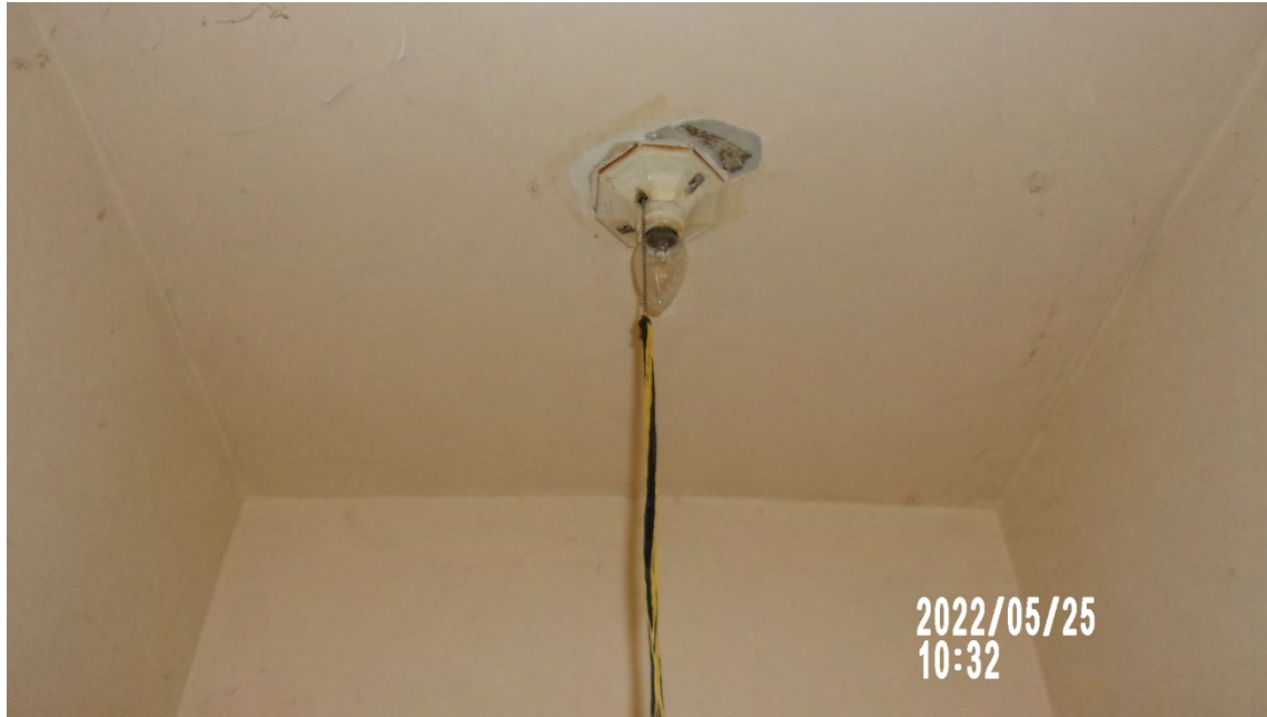
E8- Typical Light Fixture
