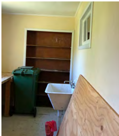
Existing plumbing in laundry room
