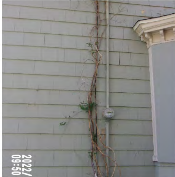
E1-Electrical Mast and Meter Base
