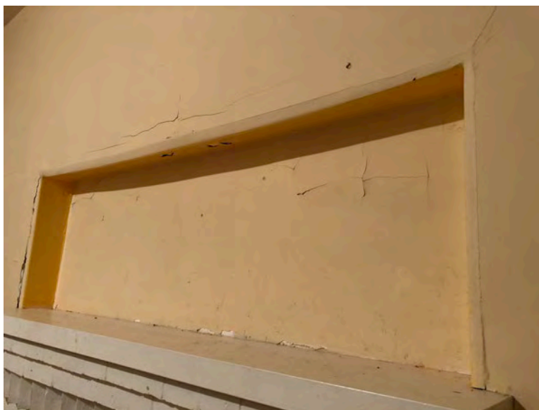
Bowing lintel in kitchen, with cracking plaster or drywall
