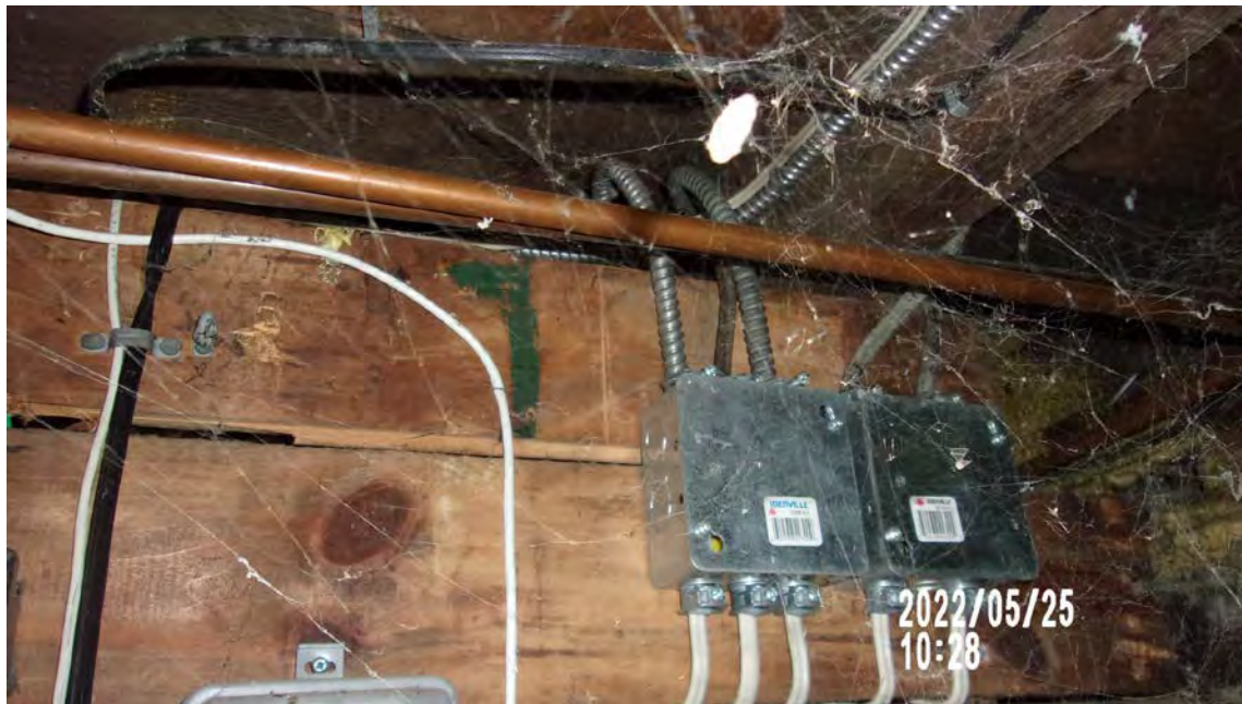
E5- Typical Wiring Methods Observed.
