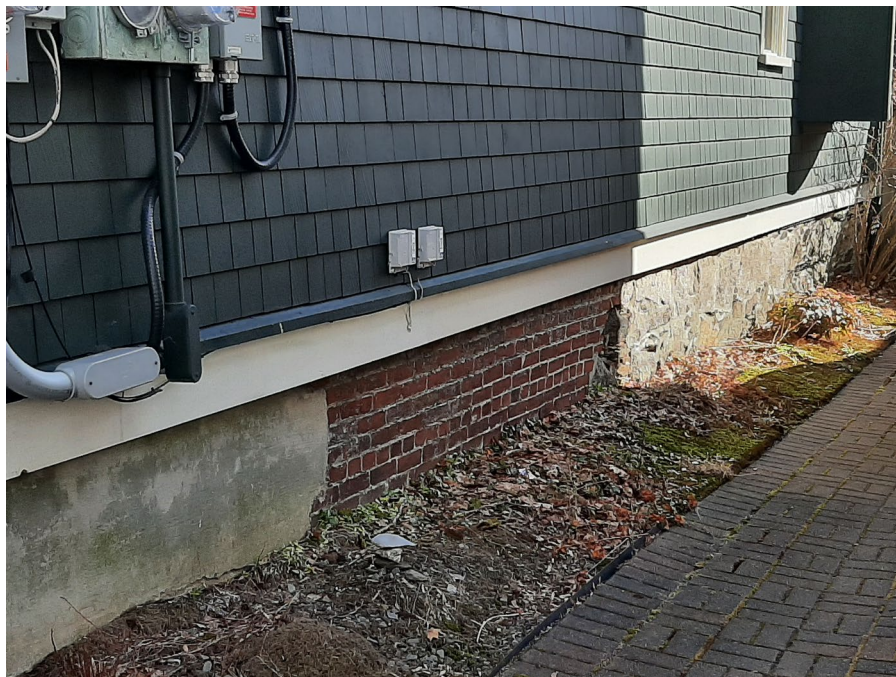
Figure 12: Foundation of 6032-6034 Charles Street, with parged concrete to the left, brick in the centre, and rubblestone and granite blocks to the right (Staff photo, 22 February 2023)
