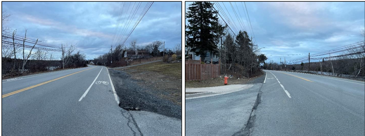
Figure 3 - View from Angler Drive looking to the north (left image) and to the south (right image)
