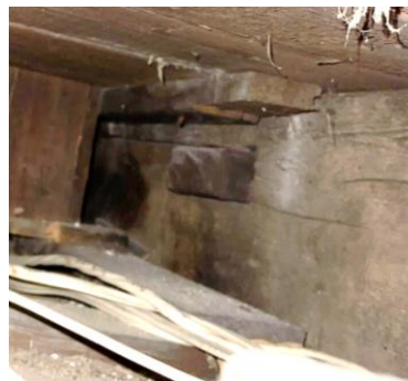
Figure 3: Photo showing the subject dwelling's timber frame construction with a mortise and tenon joint.
