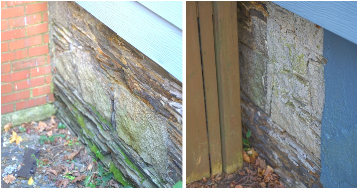
Figure 25: Detail of exposed foundations (Nov. 4, 2022)
