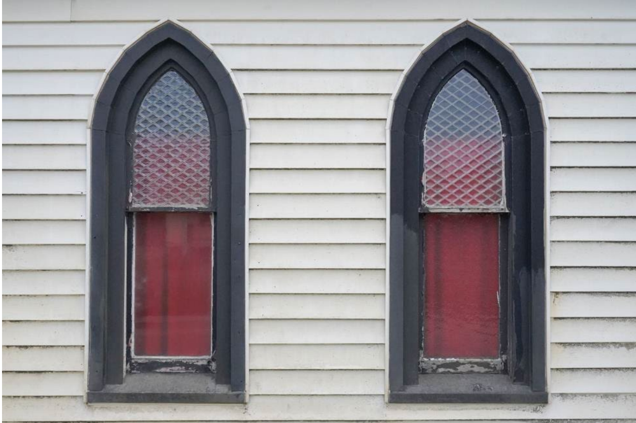
Figure 18: Two windows on the northern elevation, with upper sashes made of rolled white cathedral glass with a longitudinal diamond pattern similar to the pattern known as “quarry rolled”.(May 13, 2022)
