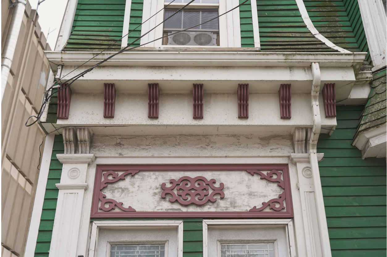
Figure 22: Detail of double cornice, pilasters, and missing transom (August 31, 2022)
