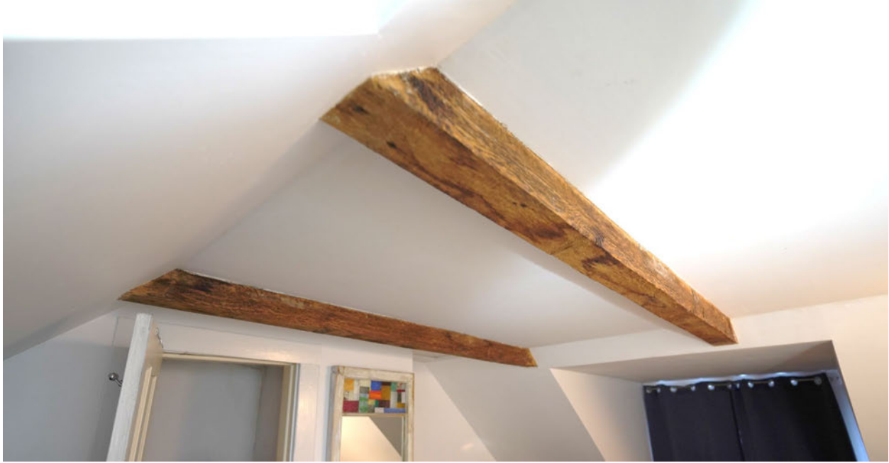
Figure 27: Photo of the very large, exposed collar ties in the upper storey of the home. (October 24, 2022)
