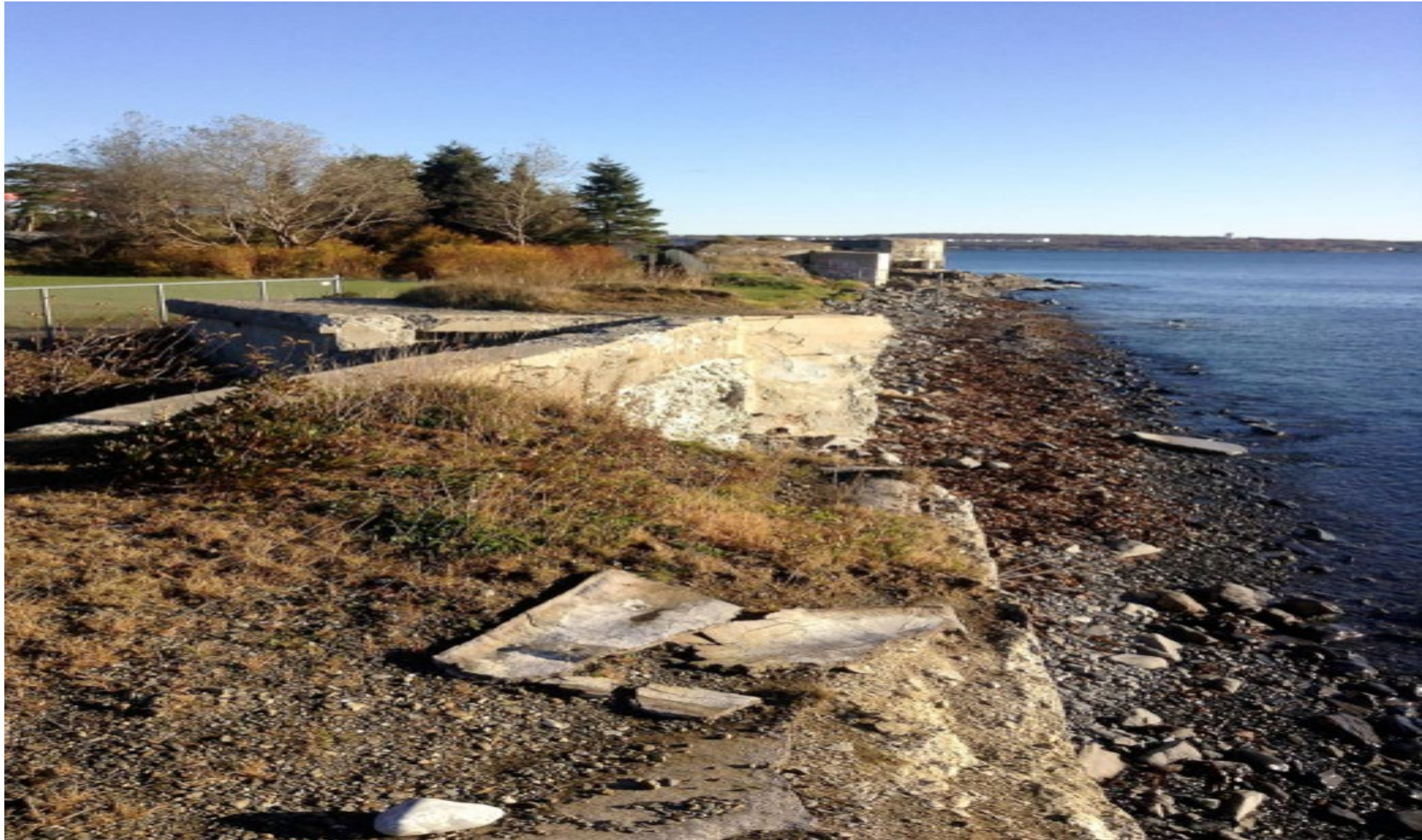
Shoreline damage to Point Pleasant Park Battery
