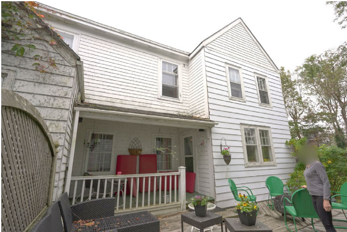
Figure 34: Eastern elevation. Note the original exterior wall of the summer kitchen, which is recessed under the upper-storey addition. (October 24, 2022)
