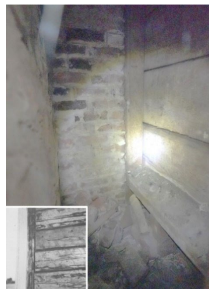
Figure 2: 6221 Coburg Road internal view of wall construction with inset photo showing another example of ‘poteaux et pièce coulissante’ construction (Oct 24, 2022)
