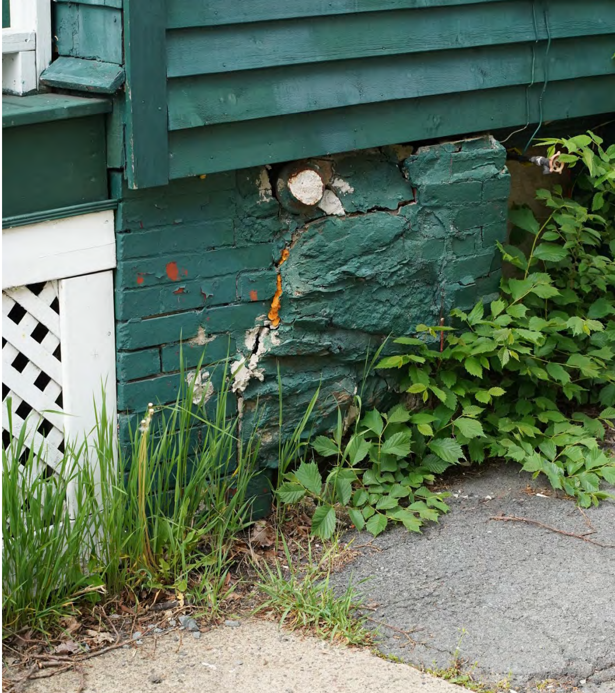
Figure 26: Condition concern with foundation (May 30, 2022).
