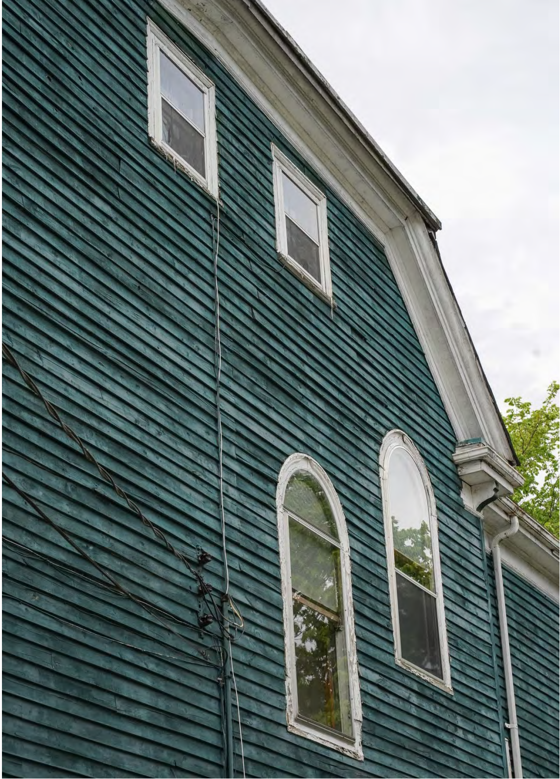
Figure 25: Condition concerns with south side windows (May 30, 2022)
