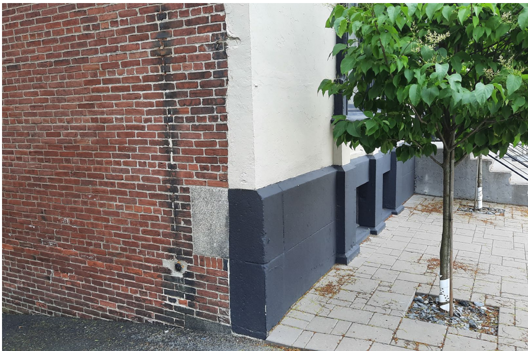
Figure 23: Painted black granite foundation with evidence of original granite to the left (July 17, 2021)
