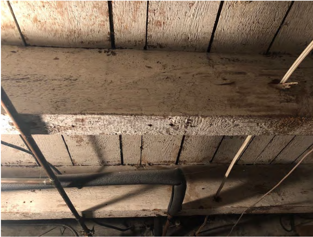
Figure 16: Milled lumber in basement of 65 Tulip Street
