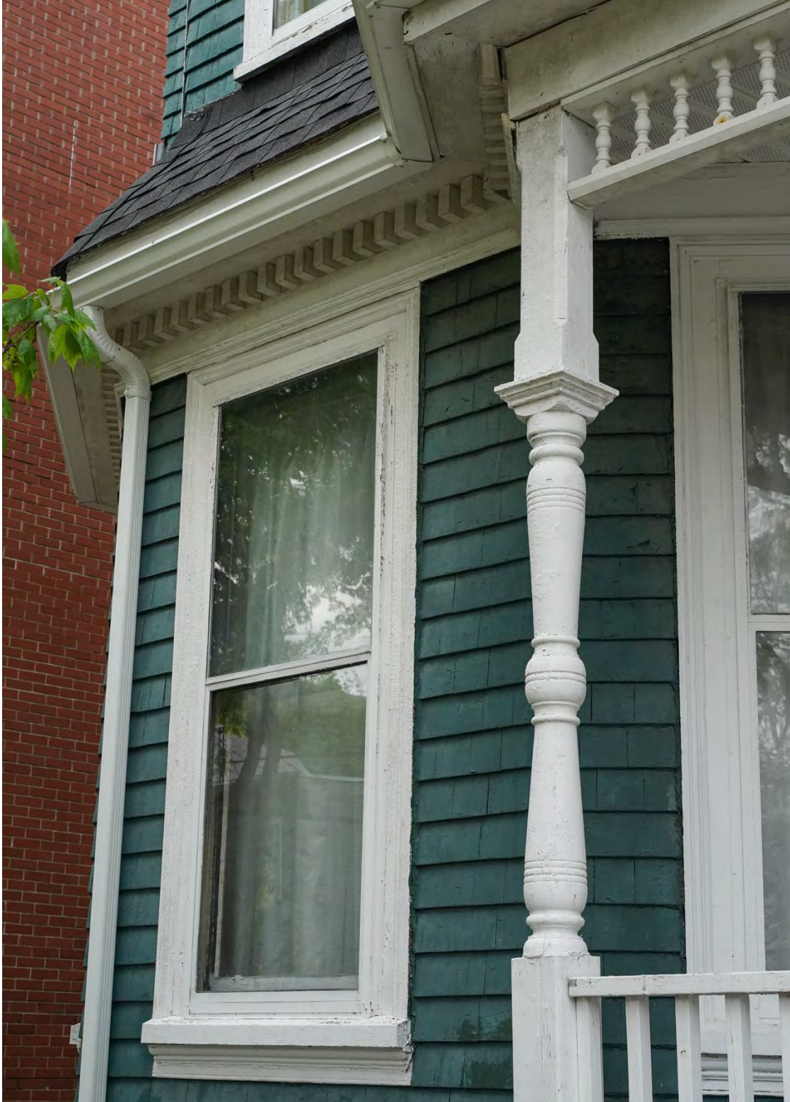
Figure 24: Detail of bay window, turned veranda post with capital, dentils, and spandrels (May 30, 2022).
