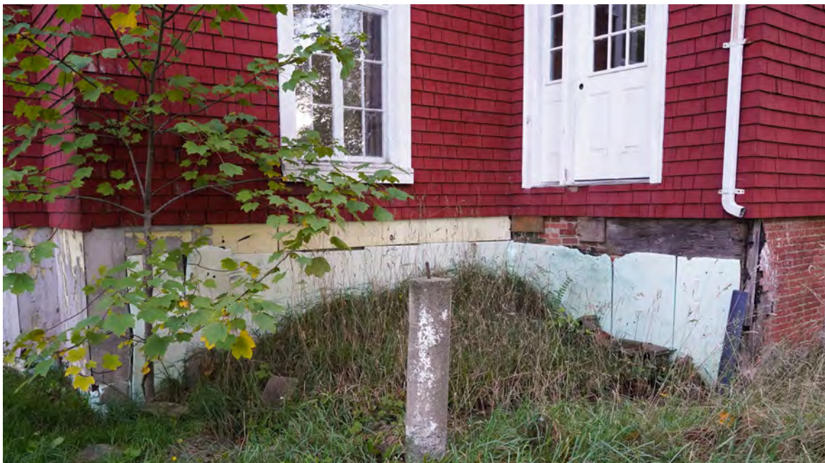
Figure 25: Detail view of foundation damage to northwestern corner of 144 Pleasant Street (October 19, 2021)
