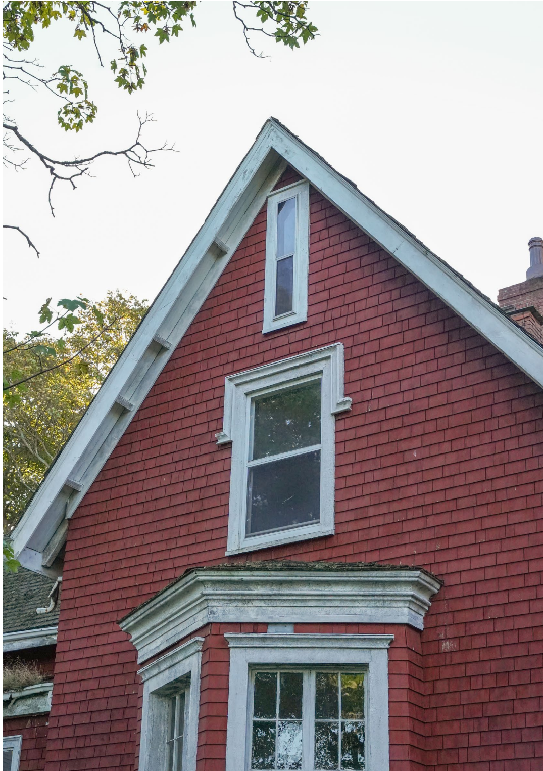
Figure 16: Detail view of northern gable, second-storey window and attic window, 144 Pleasant Street (October 19, 2021)
