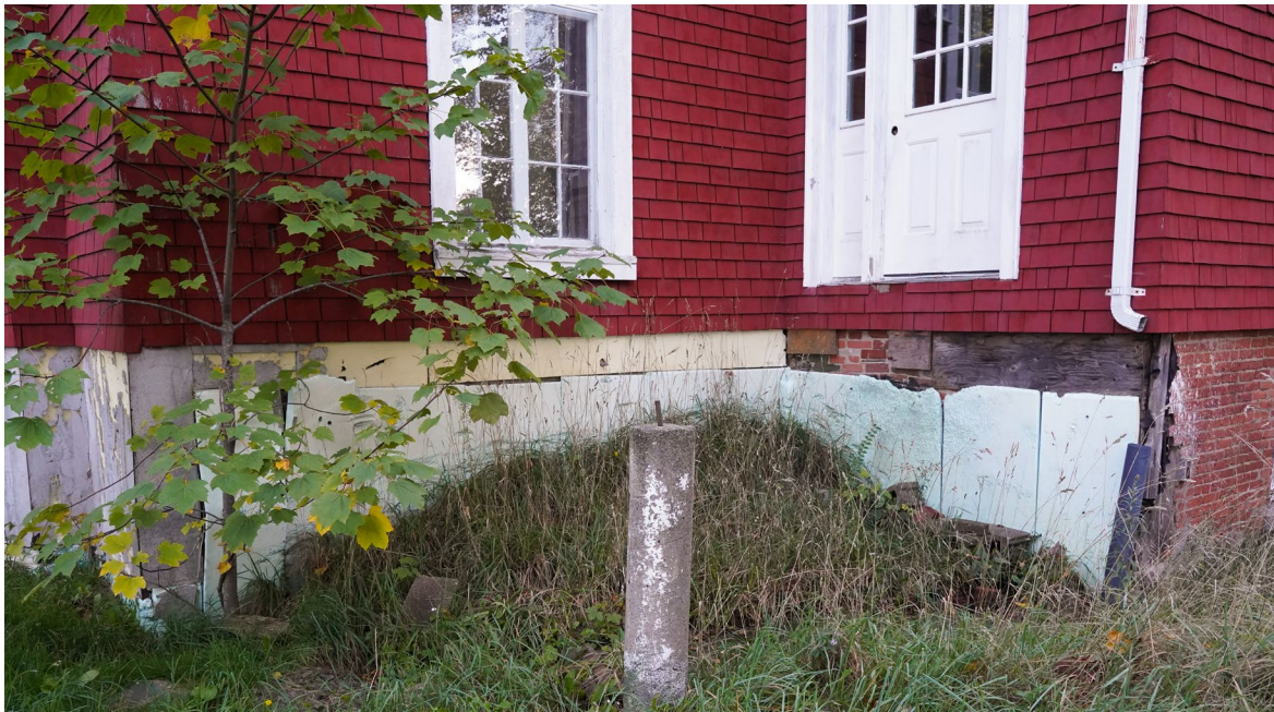
Figure 25: Detail view of foundation damage to northwestern corner of 144 Pleasant Street (October 19, 2021)
