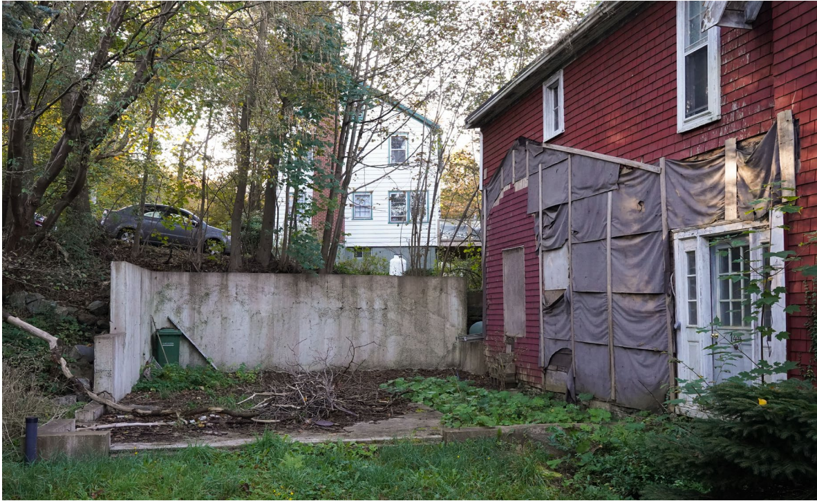
Figure 26: Detail view of foundations for the former summer kitchen/garage addition and of the eastern side of the main addition (August 30, 2021)
