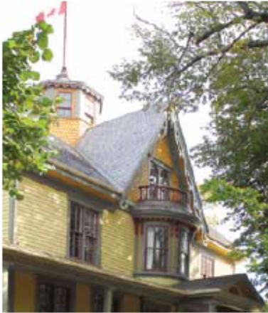
When the windows of Lefurgey House in Summerside, PEI were damaged in a fire, instead of replacing the entire windows, only the broken glass was replaced. The replacement glass, salvaged from a nearby house that was replacing its windows, had similar properties and wavy appearance.
