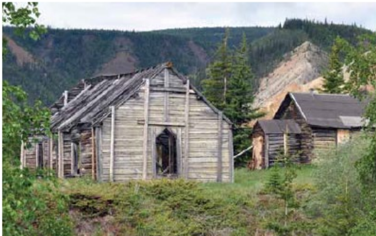
These buildings, along with others at St. Luke's Anglican Rectory and Church in the Yukon, were temporarily stabilized using a variety of measures including adding sandwich bracing, cable bracing, heavy frames, roll roofing, and covering door and window openings in order to keep out snow and rain. Stabilization allows the structures to be adequately researched and their eventual restoration to be planned.
