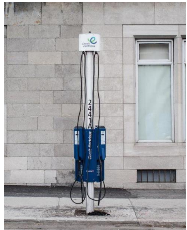
Figure 4 — On-street level 2 charging in Montreal, Quebec
