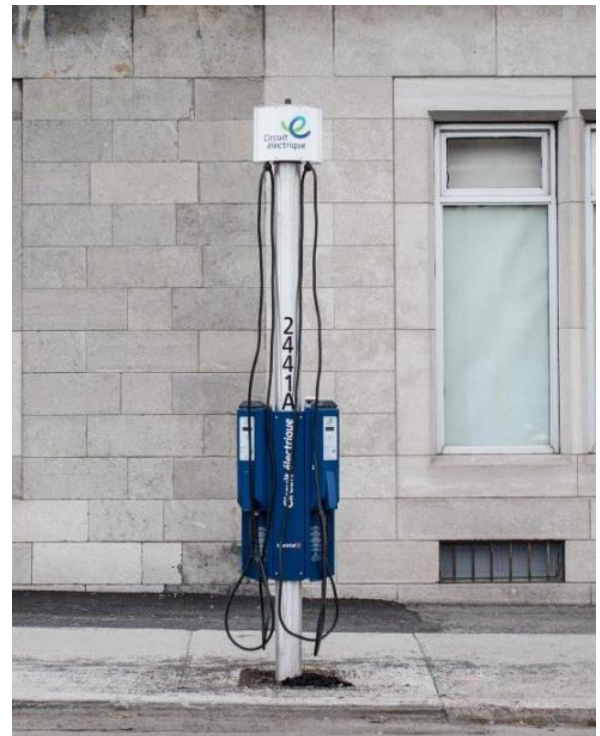
Figure 4 — On-street level 2 charging in Montreal, Quebec
